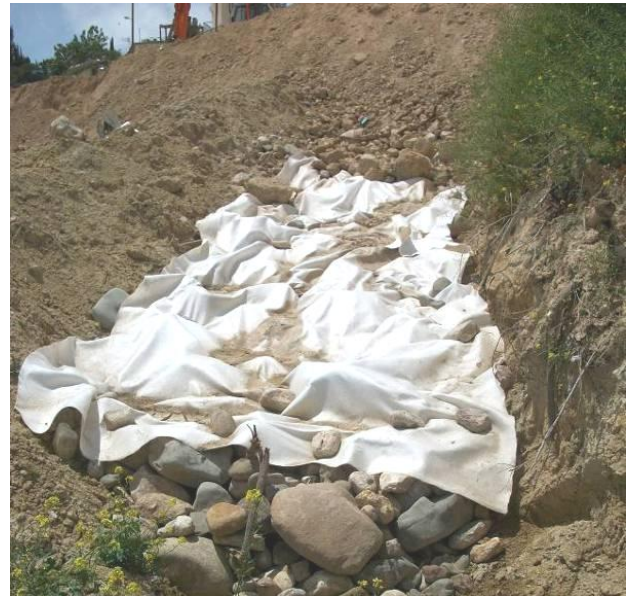
Figure 21. Trench drains filled with cobles wrapped in geotextile filter collect and dispose the groundwater.
