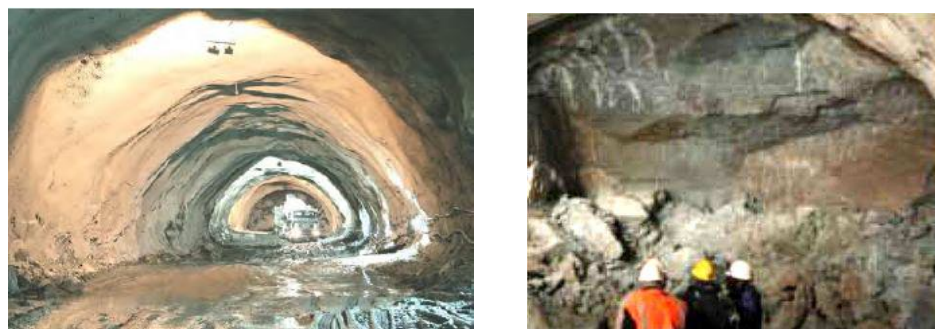
Figure 16. Response of molassic rocks during tunnelling of the “Egnatia odos” tunnels. Left: Structurally controlled overexcavation - Ag.Paraskevi tunnel (after Dounias et al 2010). Right: structurally controlled instability at tunnel face in thick sandstone layers separated by sparse thin siltstone intercalations (after Marinos et al. 2013)
