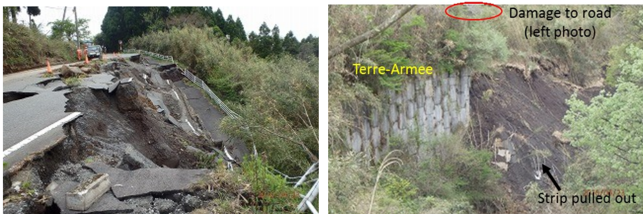
Figure 35. Damage to road embankment and reinforced retaining wall (Terre-Armee) (site 22 in Fig. 26) ( 32^{\circ} 52'52.01''N , 131^{\circ} 00'14.84''E ).
