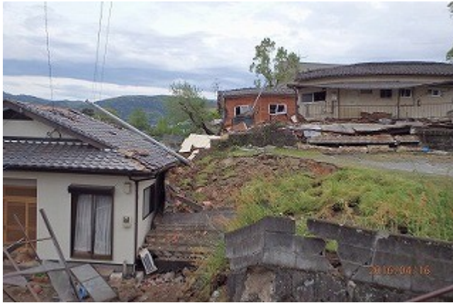
Figure 16. Ground displacement-induced damage to a residential house (Site 8 in Fig. 12) ( 32^{\circ} 47'24.96''N , 130^{\circ} 49'12.75''E ).
