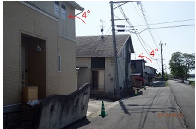
Figure 5. Liquefaction-induced damage to residential houses in Majima district (Site 2 in Fig. 3) ( 32^{\circ} 45'52.69''N , 130^{\circ} 46'7.49''E ).
