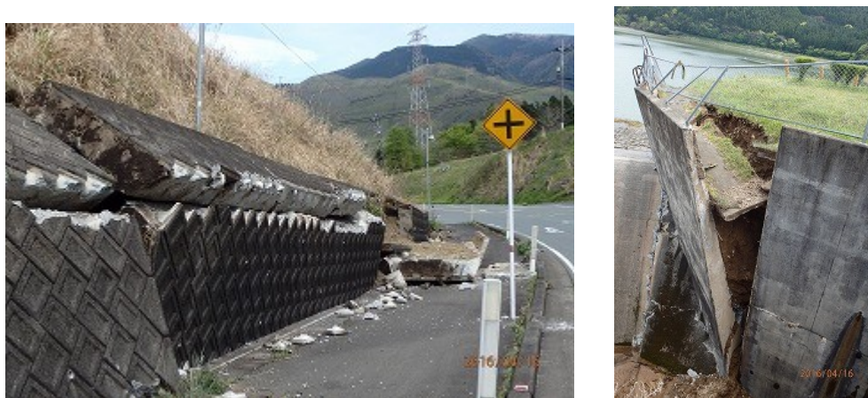
Figure 20. Damage to retaining wall and spillway retaining wall (site 12 in Fig. 12) ( 32^{\circ}50'29.22''N , 130^{\circ}55'55.83''E ).
