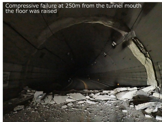
Figure 25. Tawarayama tunnel suffered from axial compression failure (Site 16 in Fig. 12) ( 32^{\circ} 51'35.68''N , 130^{\circ} 58'6.86''E ).
