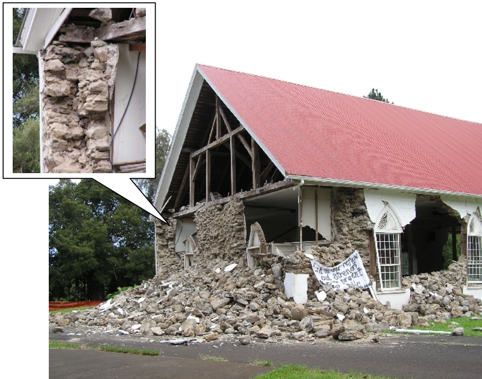
Figure 42. Location 21, Kalāhikiola Congregational Church, Kapa 'au. Weakly cemented stacked rock walls (inset) failed dramatically.
