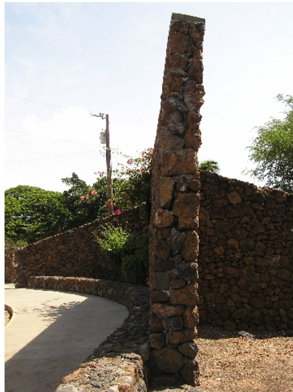
Figure 43. Location 30, Spencer Beach Park, south of Kawaihae. Apparent earthquake damage of partially mortared rock wall: wall is bent.
