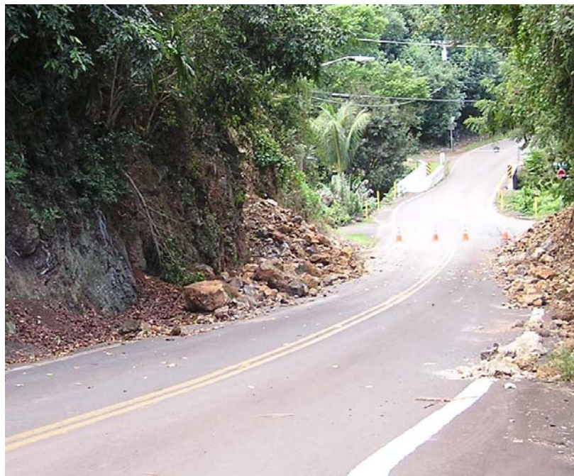
Figure 7. Hwy 270, Station 18, near Kēōkea Bay Beach Park access road. Highway was blocked by rock falls after the earthquakes.
