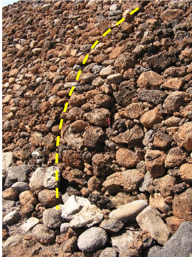
Figure 53. Location 29, NE corner Pu'ukoholā Heiau. Bulging of rock face approaches 90 degree inclination as indicated by yellow line. Bulge is clearly seen in 3-D stereo versions of Figure 54 and Figure 55.
