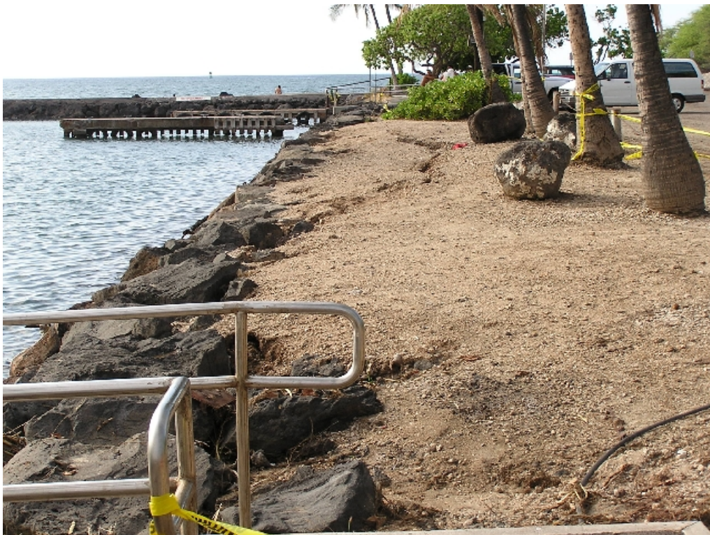
Figure 37. Location 27, Kawaihae Small Boat Harbor, showing arcuate ground crack resulting from lateral spreading.
