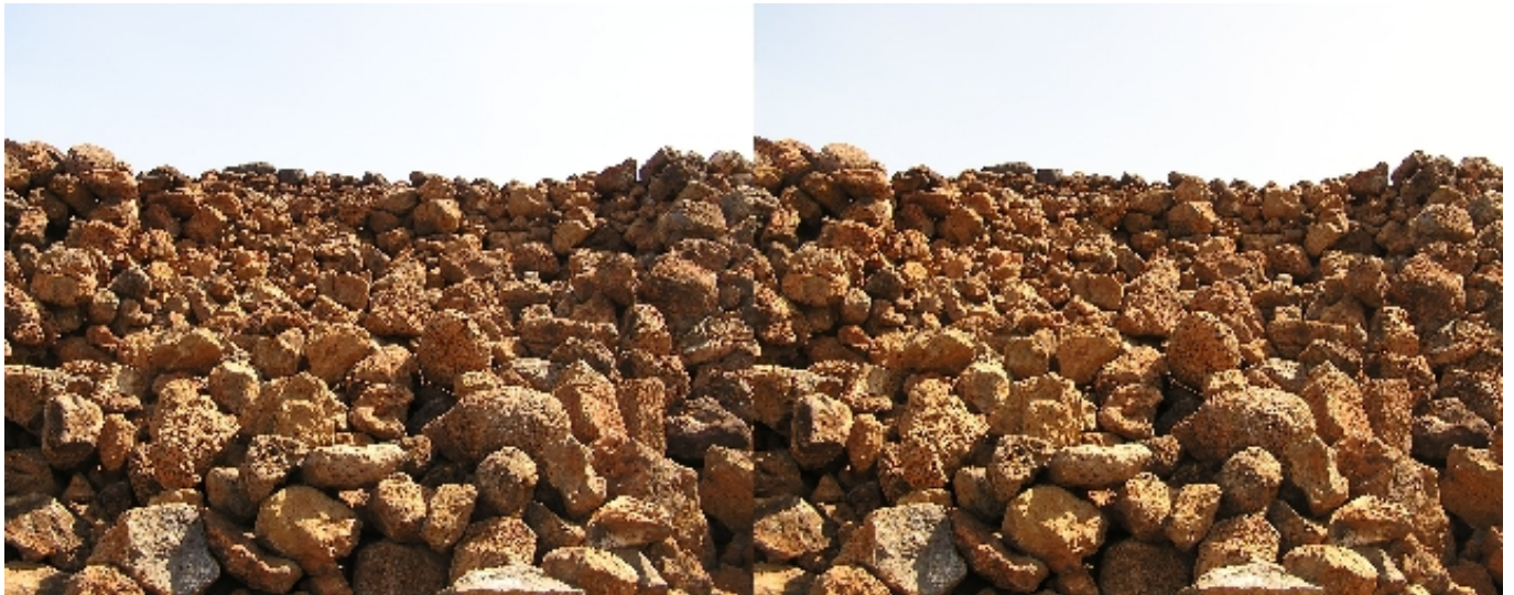
Figure 58. Location 29, slump failure in high rock wall of Pu'ukoholā heiau, west side. Stereo pair 3-D version of Figure 57.
