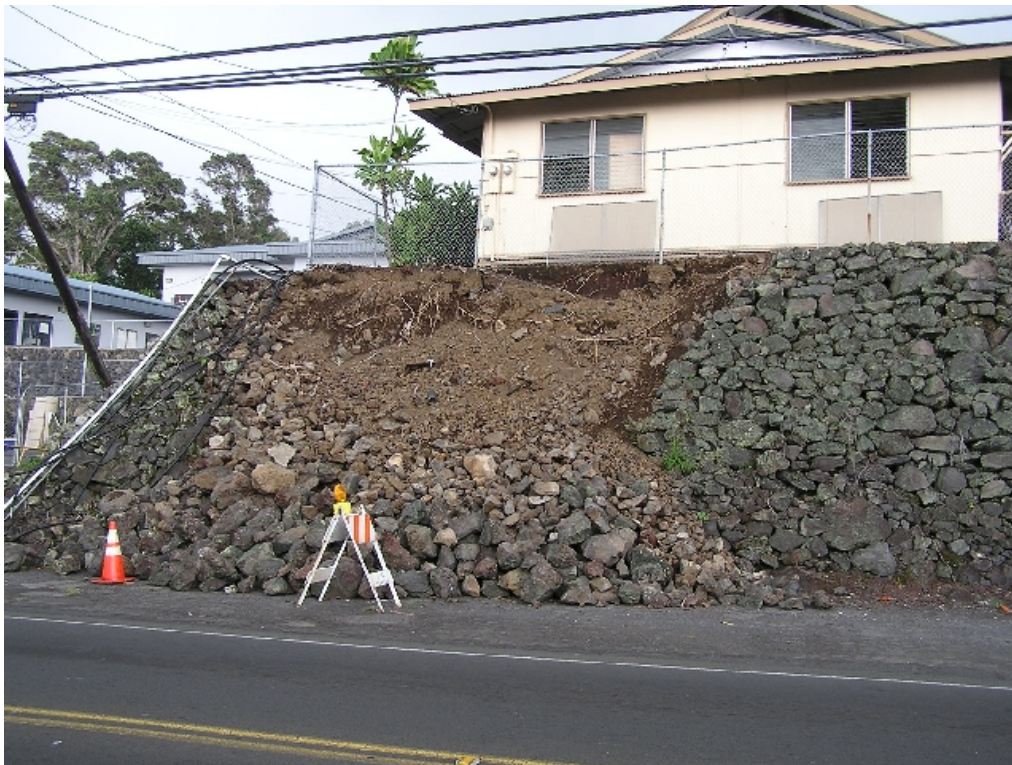
Figure 44. Location 35, Captain Cook. Failed stacked rock retaining wall. 3
