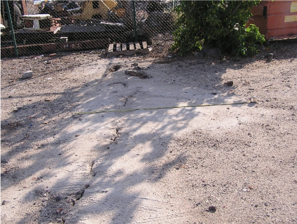
Figure 39. Location 27, Kawaihae Small Boat Harbor parking lot, adjacent boat yard at south side. Liquefied (white) sand was ejected from wide ground crack during the earthquake shaking.
