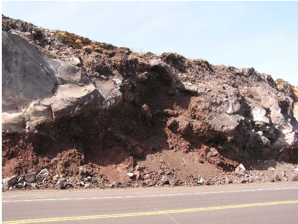
Figure 11. Location 32, Hwy 11. Failure of massive basalt blocks overlying weaker rock (weathered a'a clinker and baked zone).
