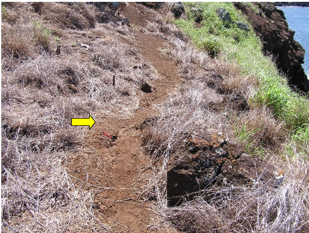
Figure 35. Location 23, Ala Kuakini Trail. Tension cracks behind cliff top (arrowed) in foreground.
