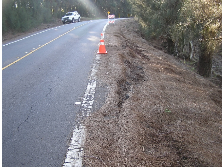
Figure 62. Location 15, north of Mile Post 9.4 Hwy 250. Slump failure of embankment on down slope side of road.
