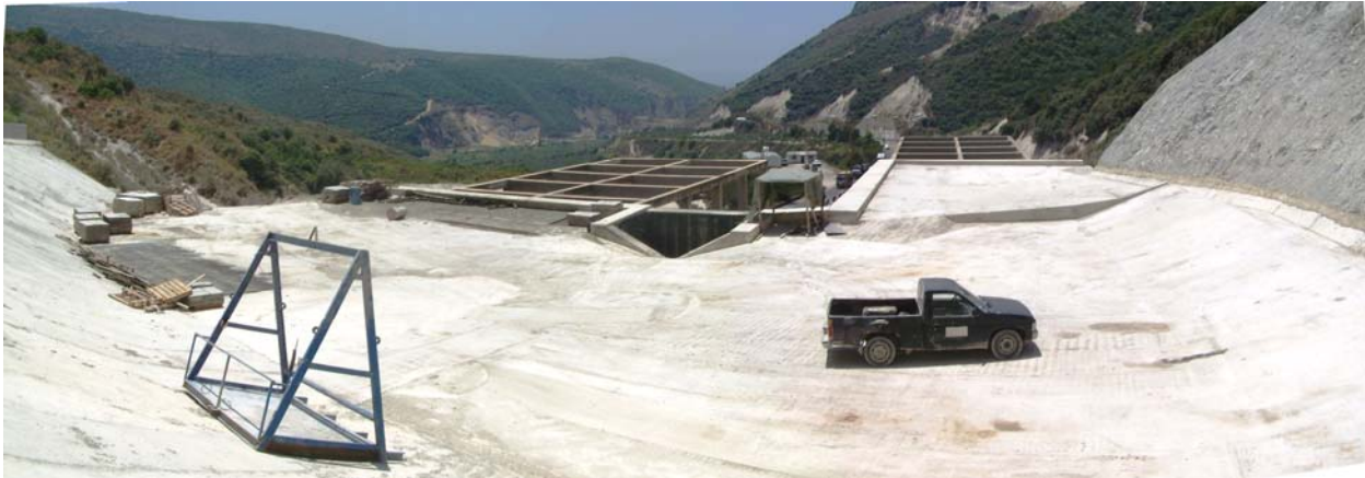
Figure 16. Regraded and Remediated Area Above the Portals and Southern Entrance/exit of Tunnels.
