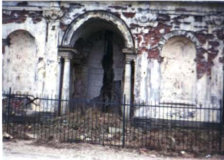
Figure 7a. Dilapidated structures of the palace: grotto.
