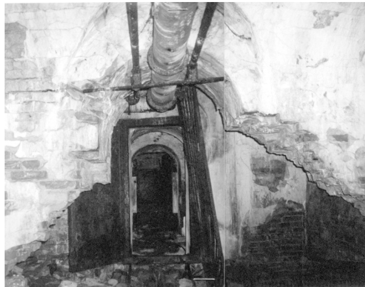
Figure 7b. Dilapidated structures of the palace: transverse walls.
