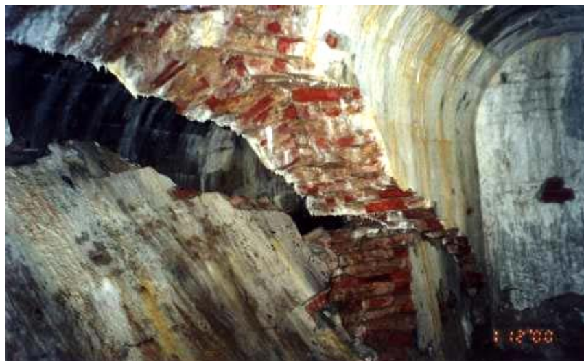
Figure 10. Collapsing cellar wall behind east loggias.
