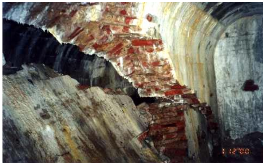
Figure 10. Collapsing cellar wall behind east loggias.
