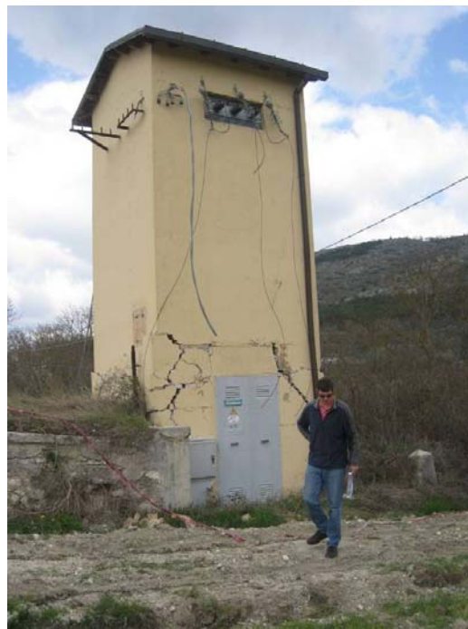
Figure 57. Heavily damaged seismometer station box (not in use at the time of the earthquake, no recording) on the northeast valley beneath the town of Castelnuovo. (42.2982°, 13.6295°).
