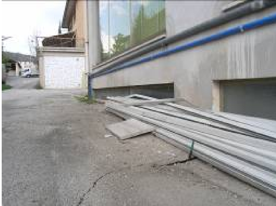
Figure 32. Ground fissures and settlement at the side of the building (42.359817°N, 13.468649°E).
