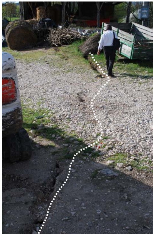
Figure 143. Ground cracks up to 1.0 m deep, 20 m long, and with maximum of 15 cm vertical displacement (down-dropped toward river) developed directly adjacent to bridge abutment (42.324N, 13.478E).
