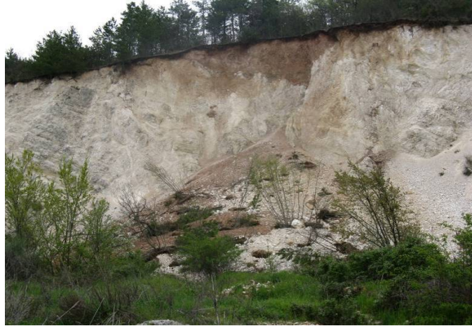
Fig. 130. Slide of a small wedge in cataclastic limestones on the SS80 at km 16.5, uphill from Arischia (42.41973N, 13.34926E).
