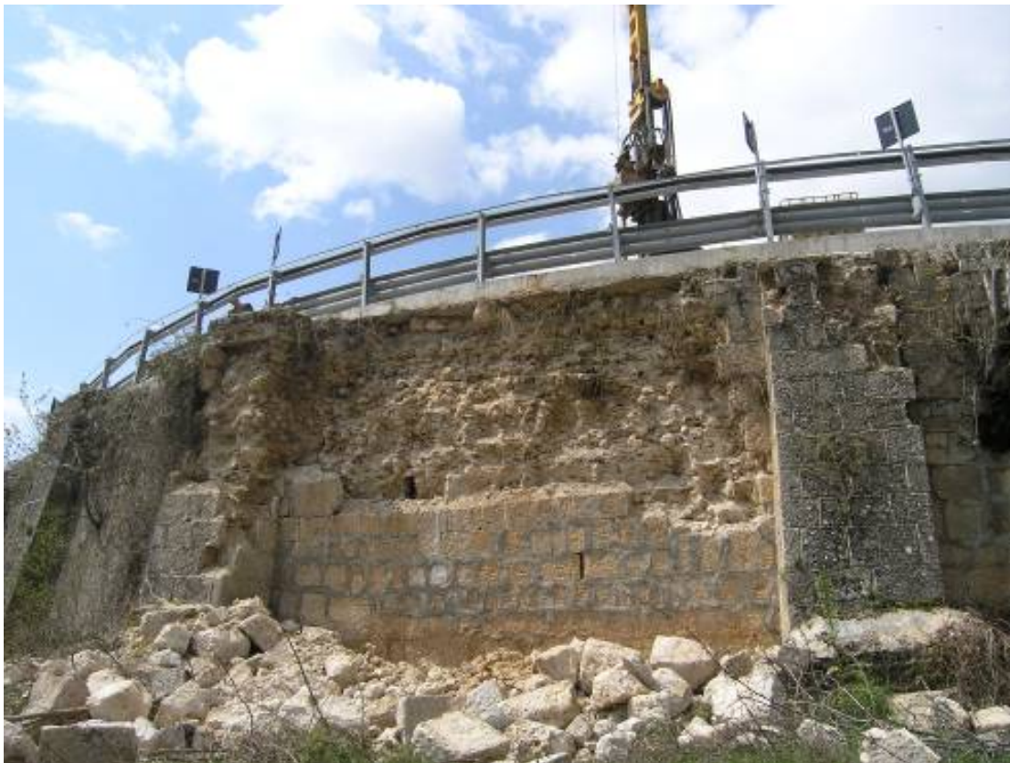
Figure 189. Partially collapsed wall at SS80 highway between L'Aquila and Campotosto ( 42.420510^{\circ}\text{N} , 13.358394^{\circ}\text{E} ).
