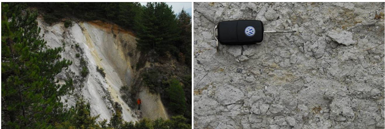
Figure 126. Cataclasite exposed along the Pettino Fault (left) and detail of cemented and interlocked particulate structure (right) (42.376N, 13.365E).
