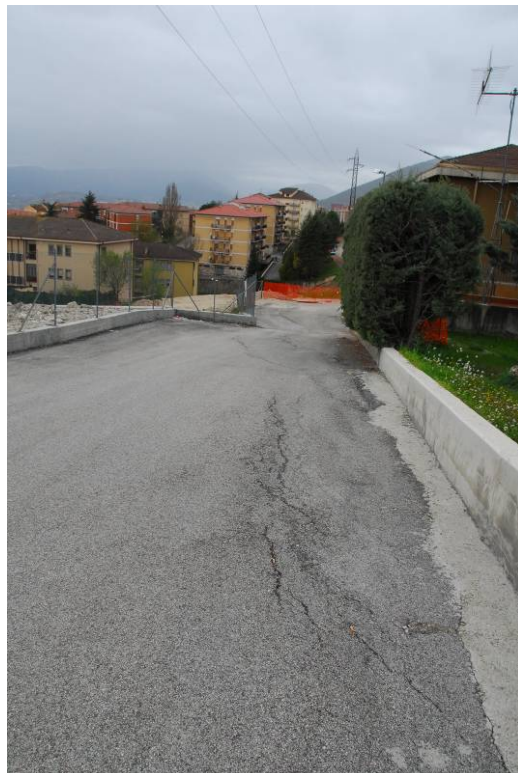
Figure 154. Cracks in the overlying asphaltic surfaces and a narrow settlement trend along the sidewall of the cut-and-cover structure (42.358N 13.415E).
