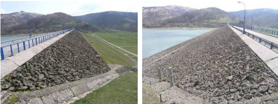
Figure 183. Downstream (left) and upstream (right) face views of Poggio Cancelli dam from the north abutment (42.558380°N, 13.338944°E).
