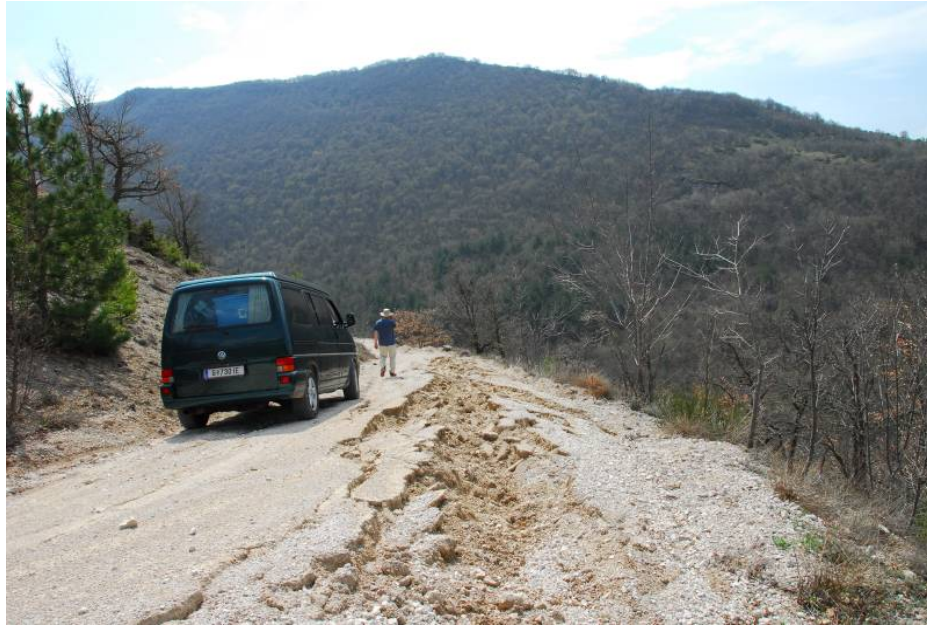
Figure 138. Failure of side-hill fill embankment (42.420N 13.376E).
