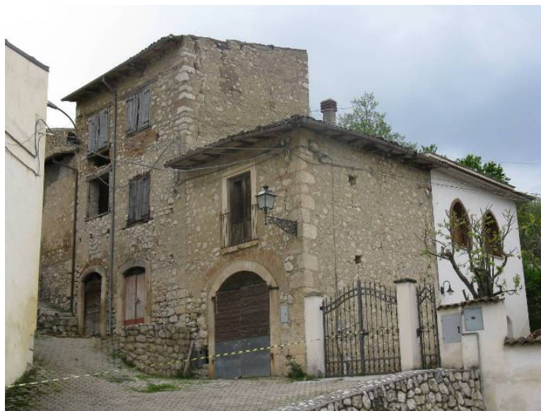
Figure 83. Casentino masonry buildings with some wall cracks.
