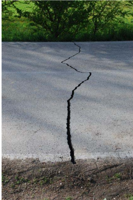
Figure 142. Typical tensile condition of road cracks, not extending into neighboring sub-base or approach fill embankment (42.324N, 13.478E).
