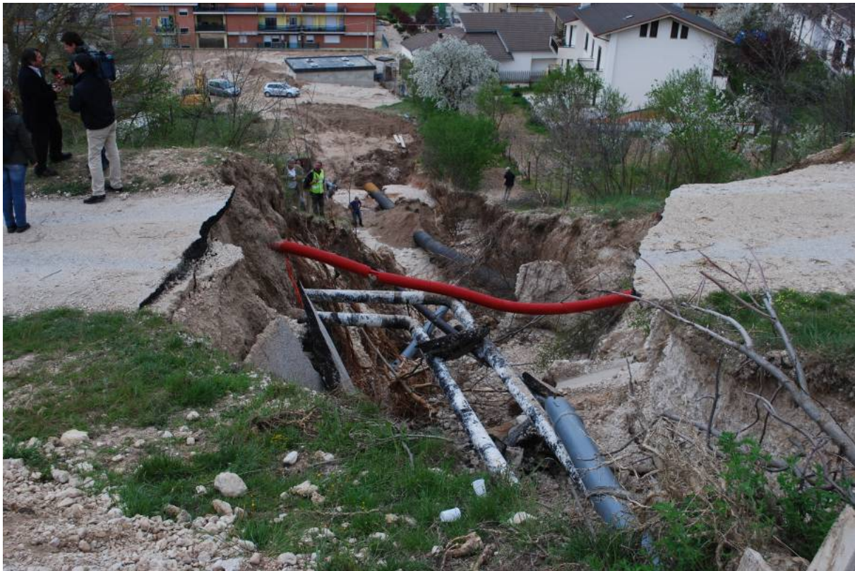
Figure 27. Paganica village: broken major water pipe (repaired) due to co-seismic rupture (Lat. 42,36537N Long. 13,46803E) (Photo by Mylonakis G).
