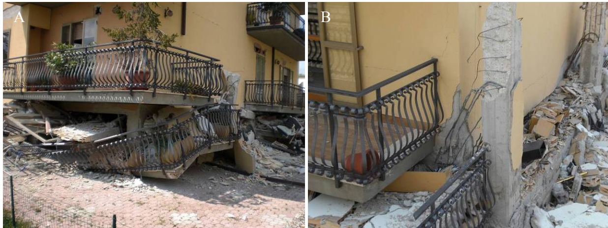
Figure 74. San Gregorio eastern part. (A) RC building “pancake” collapse, (B) Detail of sheared pillars.
