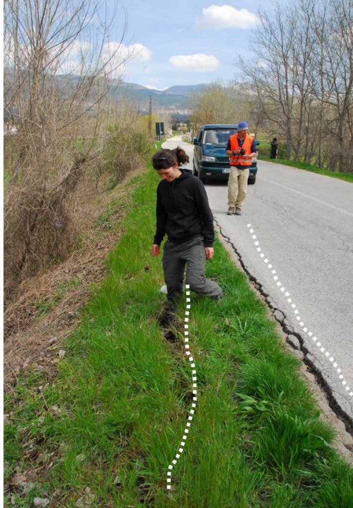
Figure 146. Approximately 15-20 cm lateral displacement of approach fill (42.325N, 13.463E).
