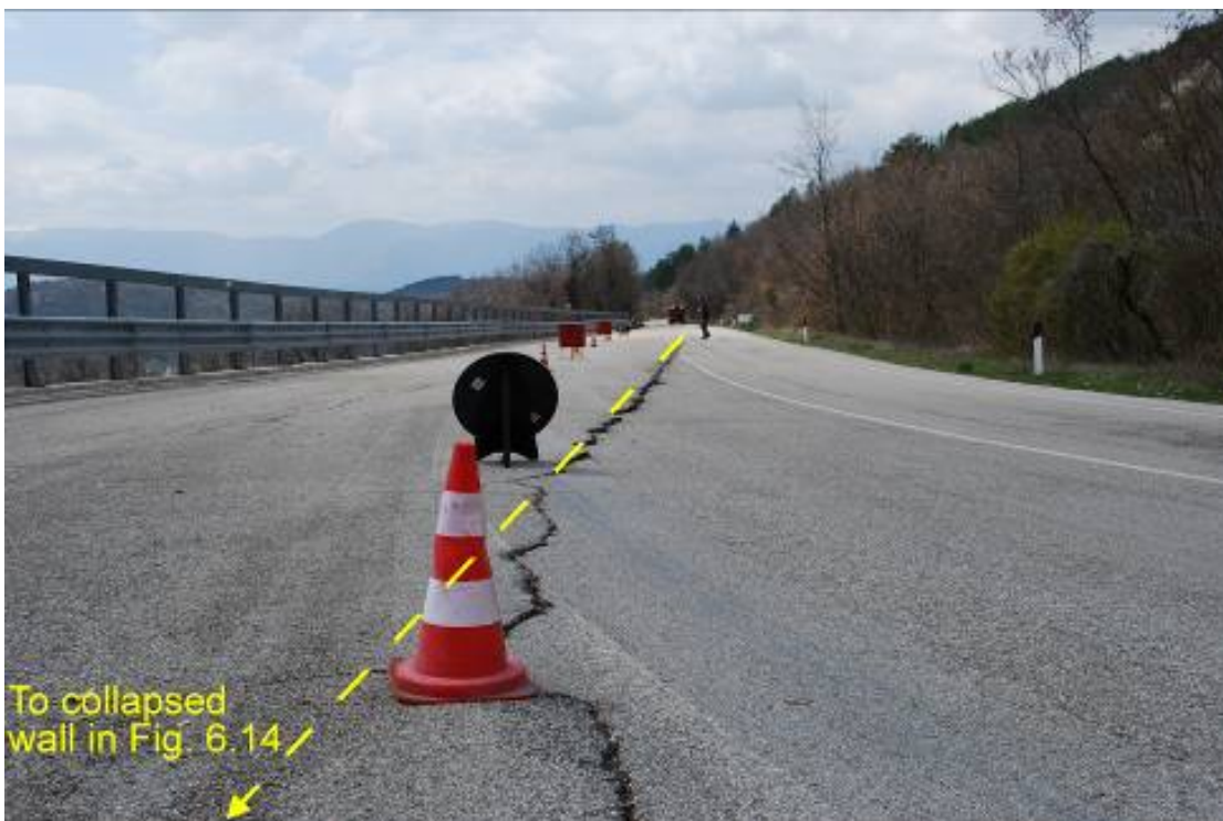
Figure 190. Pavement cracking in SS80 roadway (from L'Aquila to Campotosto) in the location of collapsed masonry retaining wall ( 42.420510^{\circ}\text{N} , 13.358394^{\circ}\text{E} ).
