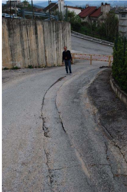
Figure 155. Seismic compression of trench backfill in the town of Paganica (42.365N, 13.465E).
