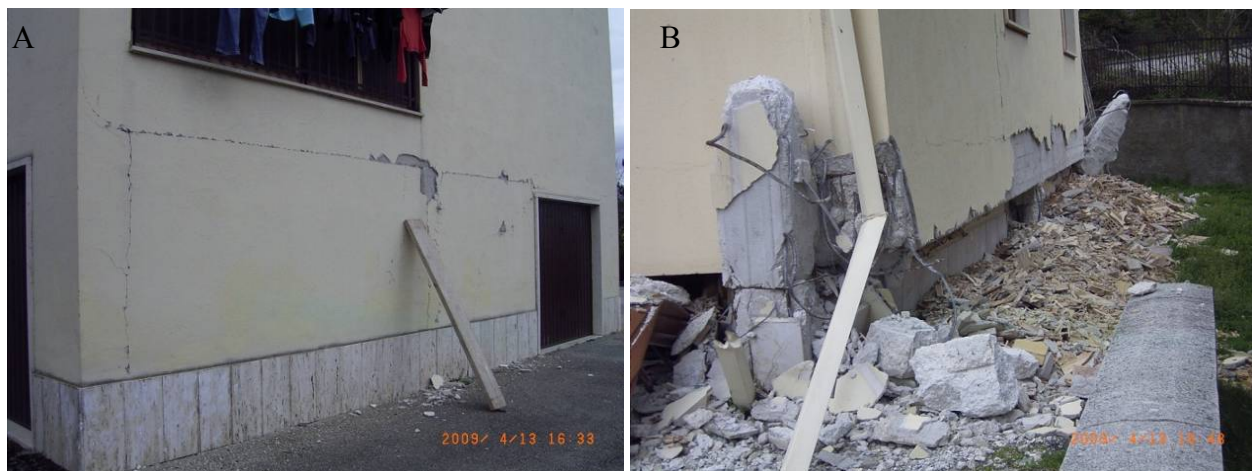
Figure 109. Damage on the structures in the cluster in zone (d). (A) Waypoint GB-22-1 (D1), (B) Waypoint GB-23-1 (D5).
