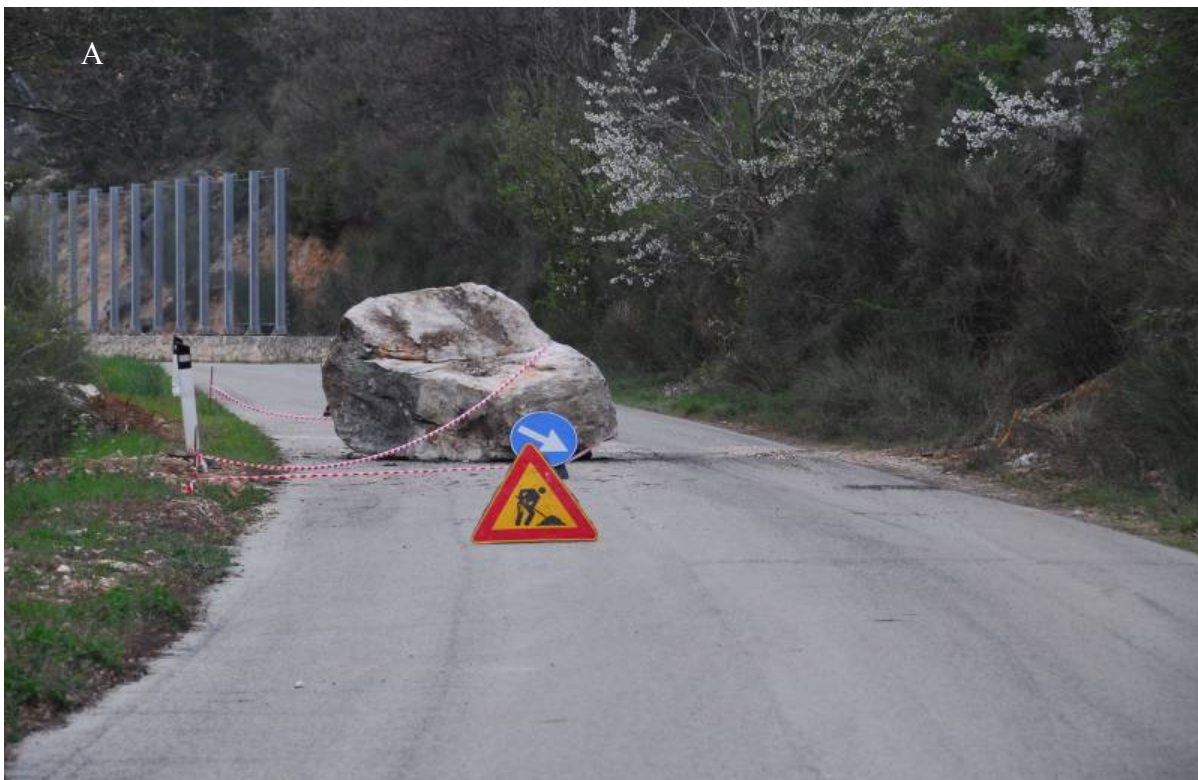
Figure 113. (A) Large block of a rock fall event (42.266N, 13.585E).
