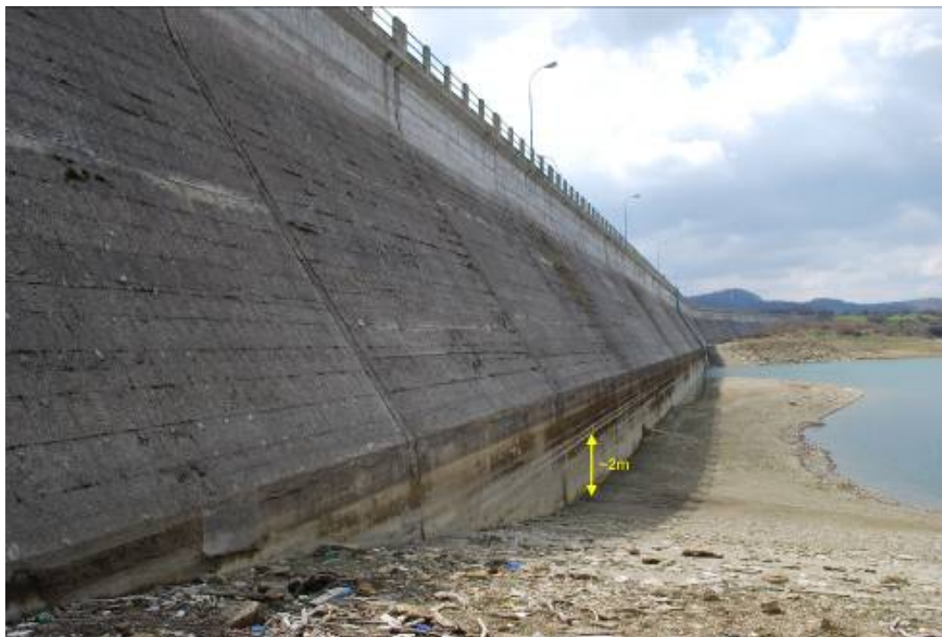
Figure 178. Upstream face of Sella Pedicate dam. The lowering of water level decided by ENEL following the main shock is evident in the photo (42.514954°N, 13.369194°E).
