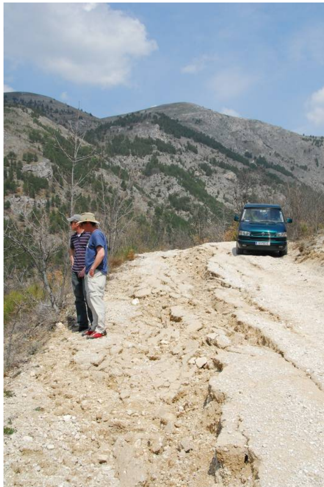
Figure 139. Failure of side-hill fill embankment (42.420N 13.376E).
