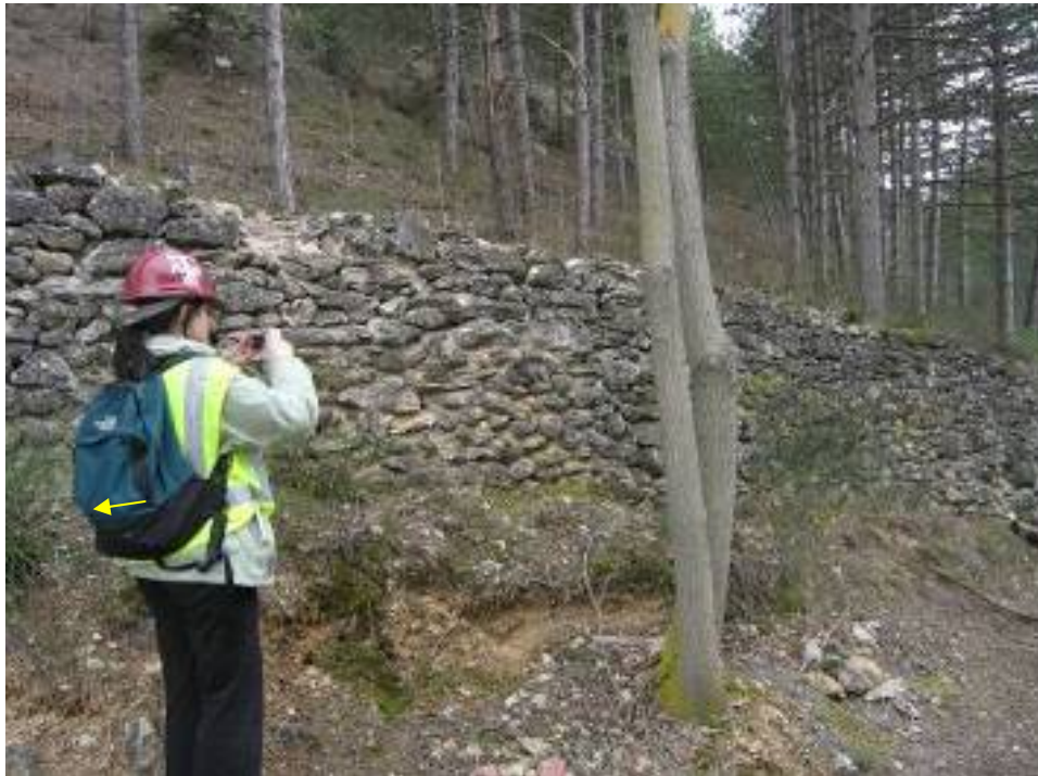
Figure 185. Minor damage on masonry wall in severely shaken Pettino area (42.374011°N, 13.367498°E).
