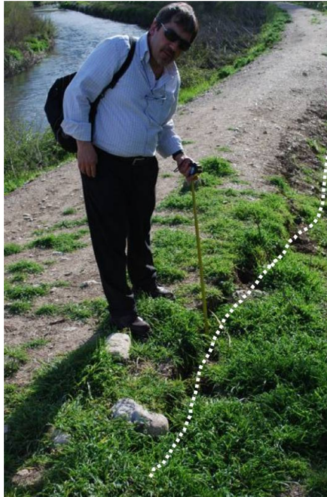
Figure 144. Ground cracks developed along levee crest adjacent to bridge abutment (42.324N, 13.478E).
