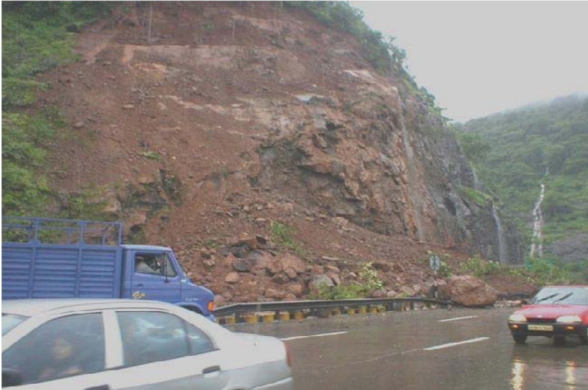
Figure 3. Rockfall and debris in 2004.
