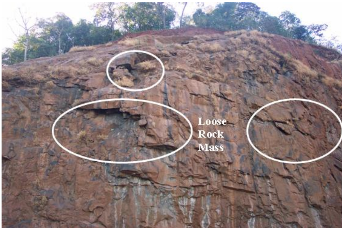
Figure 5. Vertical joints and formation of wedge along slope face.
