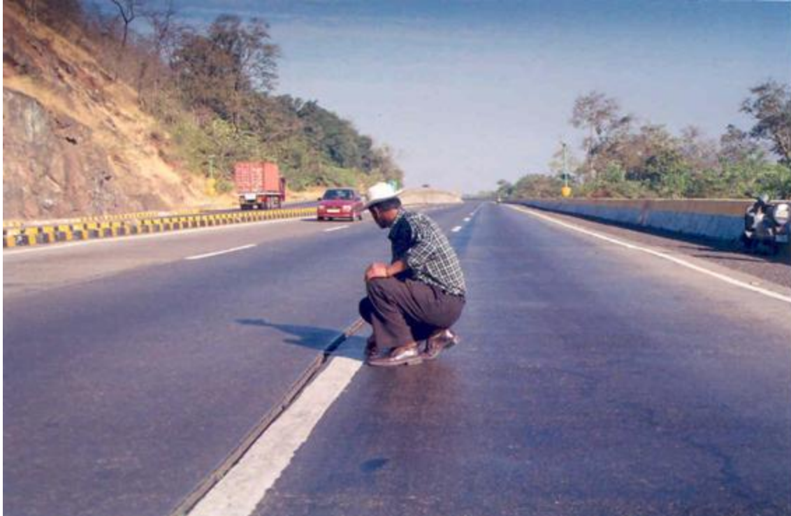
Figure 13. Dislodged rigid pavement.
