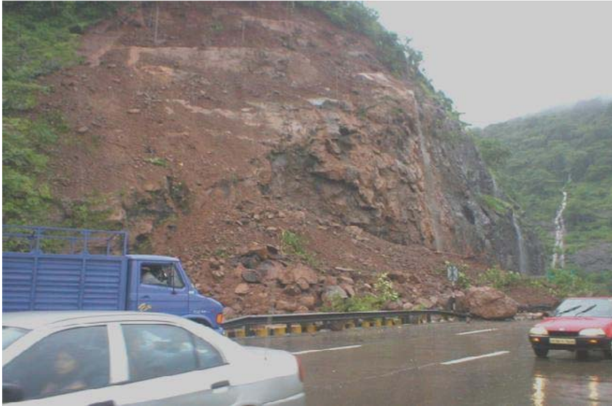
Figure 3. Rockfall and debris in 2004.
