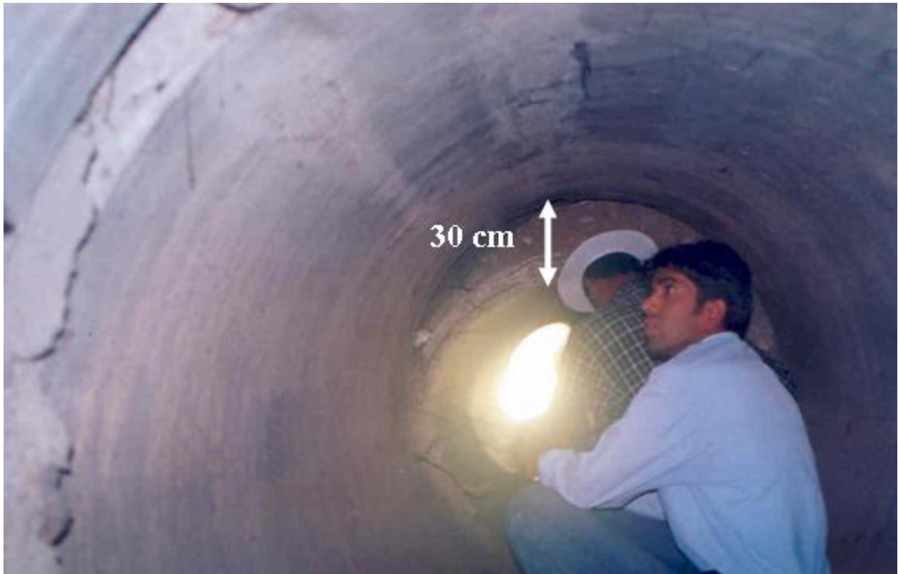
Figure 11. Dislodged pipe culvert.
