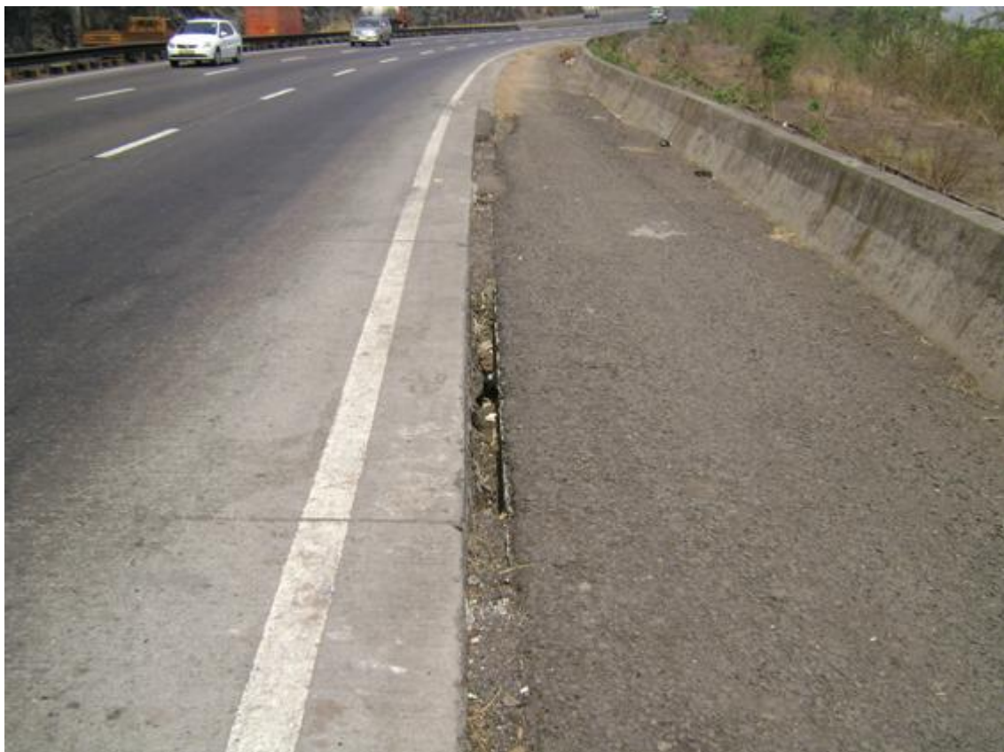
Figure 14. Crack between rigid and bituminous pavement.
