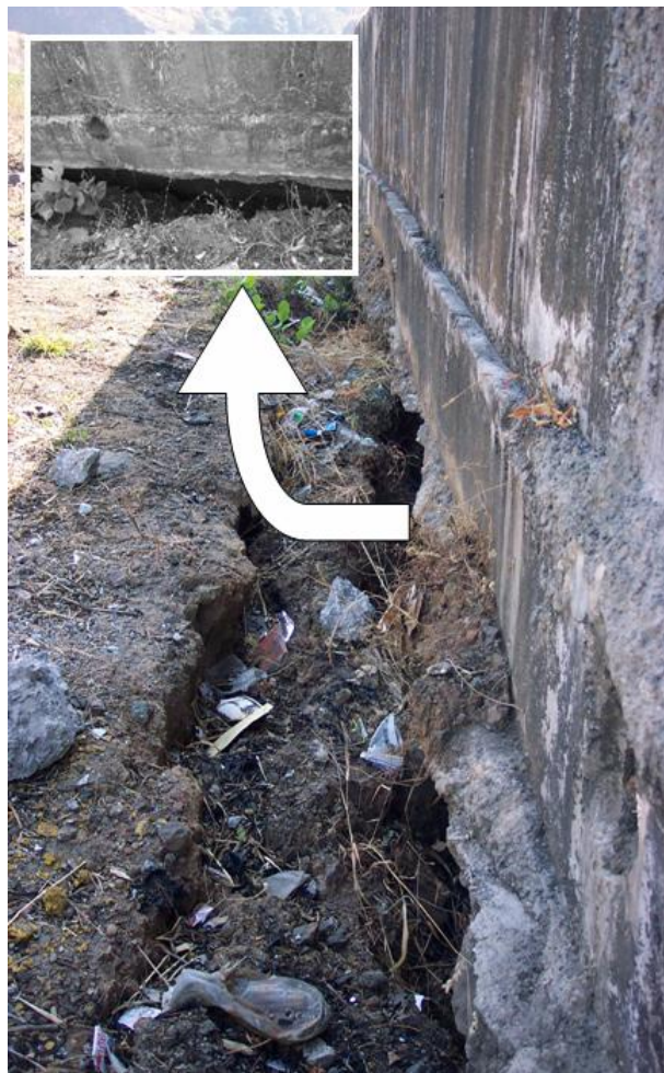
Figure 16. Embankment scoured below the crash barrier.
