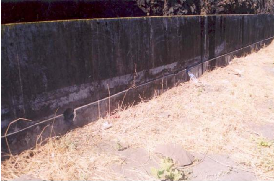
Figure 15. Drainage holes left open on embankment surface.
