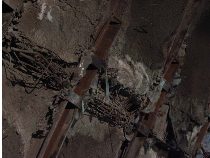
Figure 17. Detail of deformable element 6 at chainage 1443 m prior to casting of final lining.
