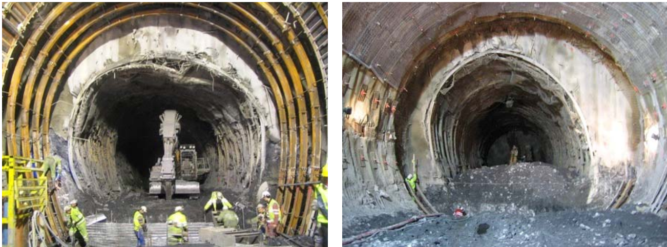
(a) (b) Figure 1. Squeezing rock reduces the tunnel cross section in the Saint Martin La Porte access adit (Lyon-Turin Base Tunnel). The photographs show re-mining works needed in order to cope with the difficult conditions encountered.
