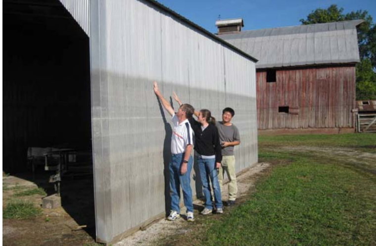
Figure 21. High water marks on barn within the Brevator levee system.
