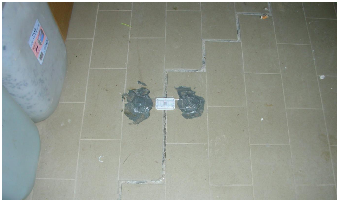
Figure 3. Floor damage inside the warehouse.
