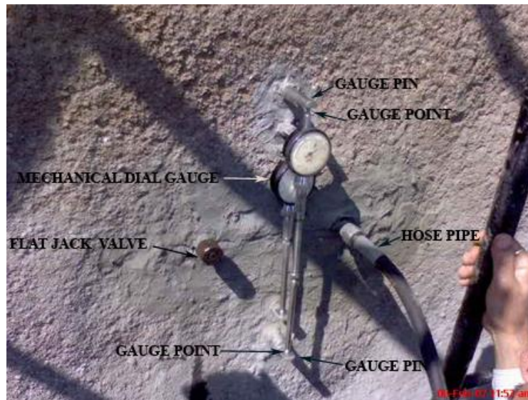
Figure 14. View of embedded flat jack and four reference pins in the slot.
