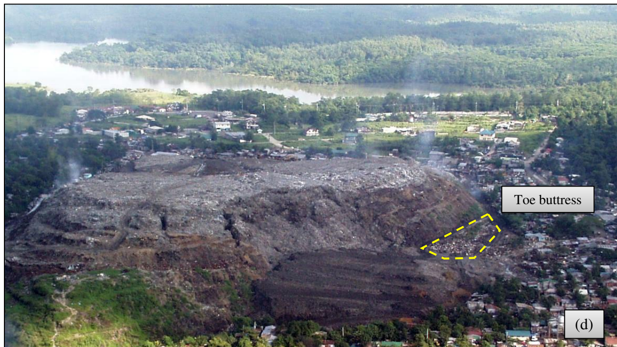
Figure 6. Slope geometry and failure surface after failure (a) evidence of seeping leachate, (b) representative slope inclination, (c) location of slope benches, (d) toe buttress (photos by S.M. Merry).
