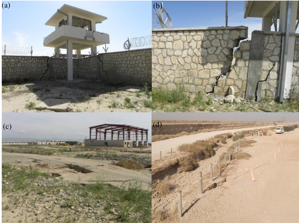
Figure 2. a. Damaged guardhouse and security wall in Kunduz, b. security wall damaged in Kunduz, c. settlement basin through a road in Kunduz, d. slope failure next to earthen drainage ditch in Mazar-e-Sharif as evidenced by coned off area.
