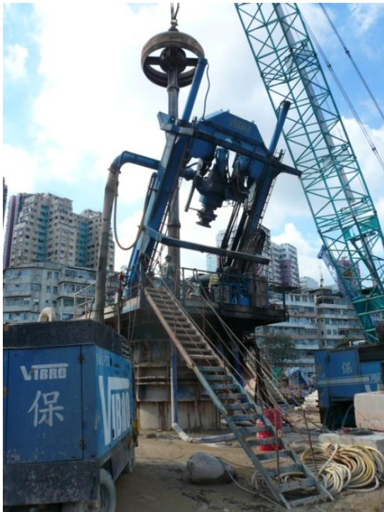
Figure 6. RCD mounted on casing top.
