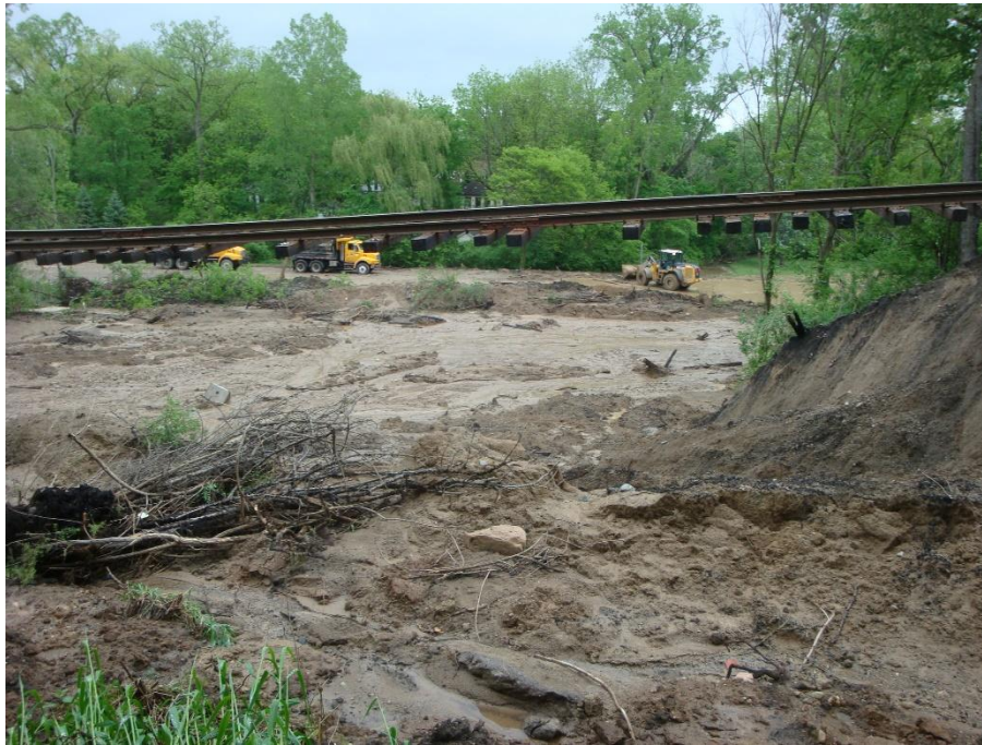
Figure 4. View of the conditions downhill of the failure showing deposition of debris and water. Trucks and dozer are operating on Plymouth Rd. and flooded area further back is a flooded public park.
