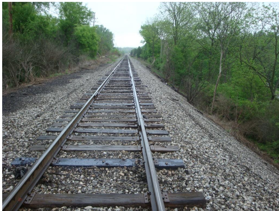
Figure 3. View of intact portion of the embankment immediately to the East of the failure area. One can see that the uphill part of the embankment (left) is supported by natural ground that is at a much higher elevation than the downhill part of the embankment (right).
