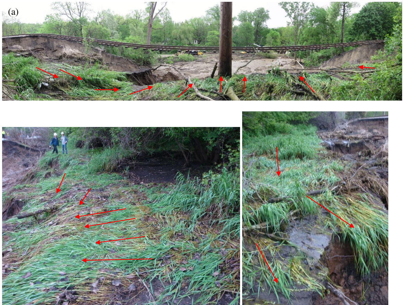
Figure 13. View of the failure and the reeds uphill of the embankment. The arrows are parallel to the direction of the fallen reeds that bent and broke during the abrupt emptying of the ponding water and fell on the ground with their orientation pointing to the initiation point of failure. (Fig. 13a by Karl Jansen, ceephotos.com)
