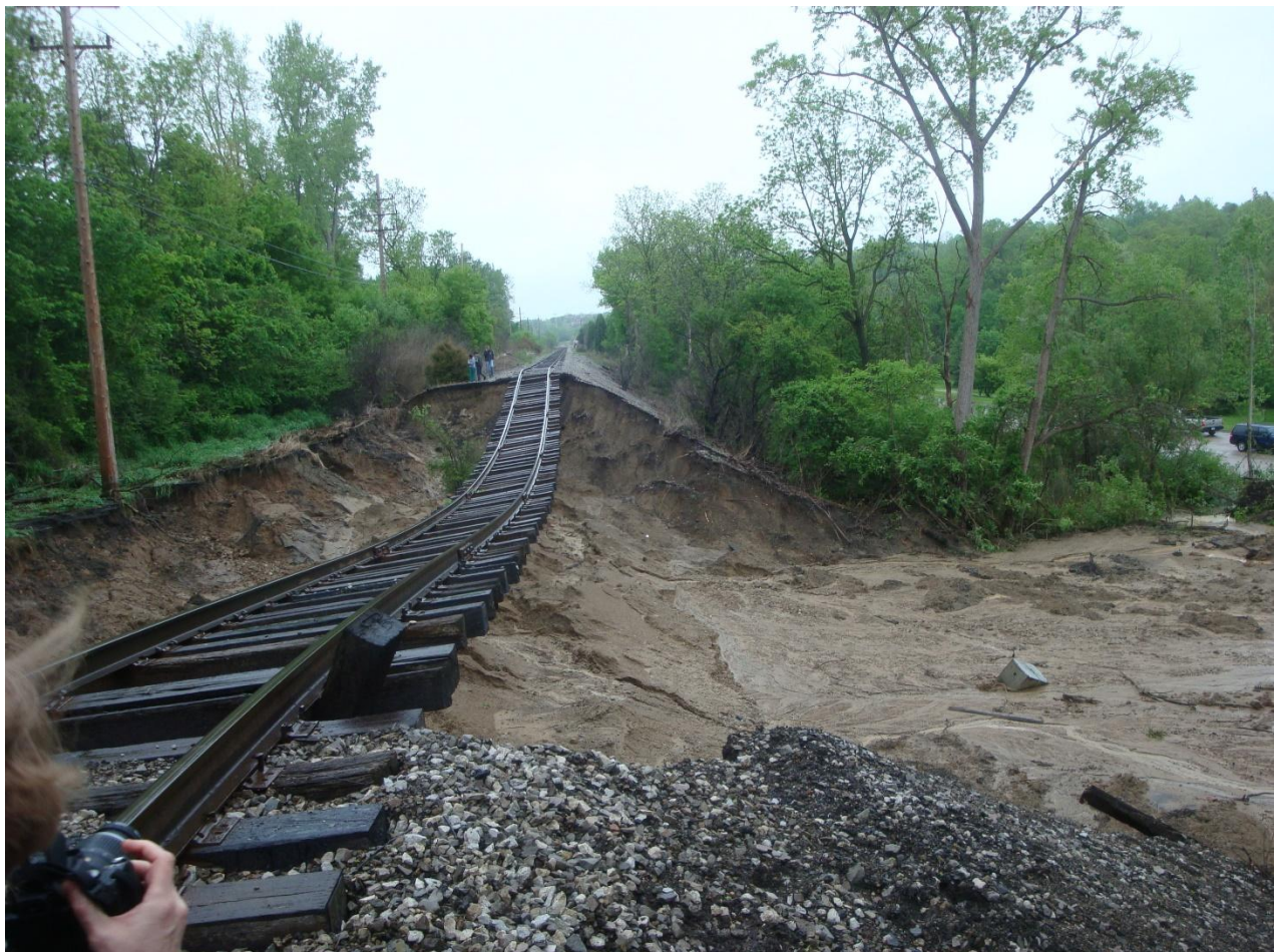
Figure 1. View of the railroad embankment failure looking East.
