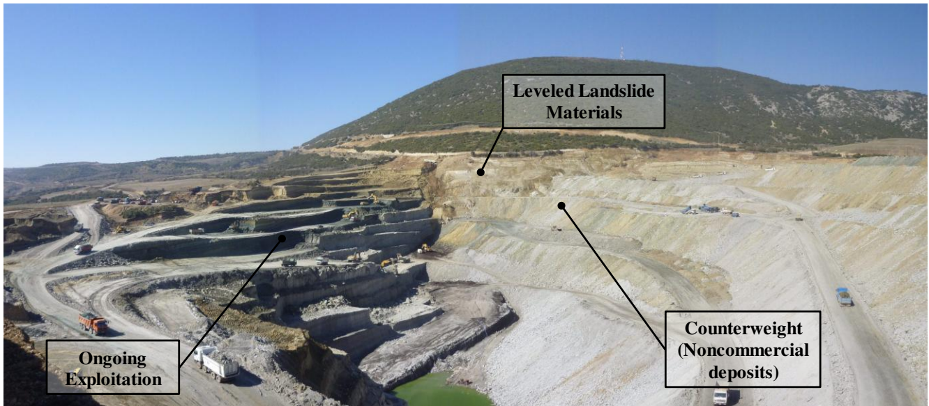
Figure 13. Aspect of the coal mine area after completion of counterweight construction and leveling works (March 2012).
