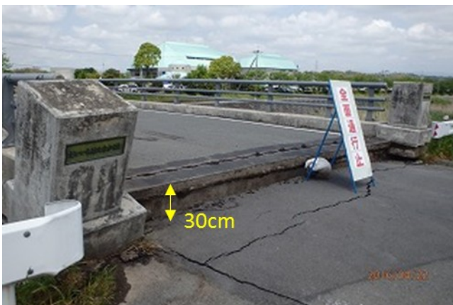
Figure 8. A large gap at bridge girder due to settlement of embankment (Site 4 in Fig. 3) ( 32^{\circ} 47'2.15''N , 130^{\circ} 49'17.70''E ).
