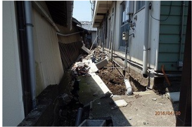
Figure 17. Ground displacement-induced damage to a residential house (Site 9 in Fig. 12) ( 32^{\circ} 47'14.48''N , 130^{\circ} 48'41.06''E ).
