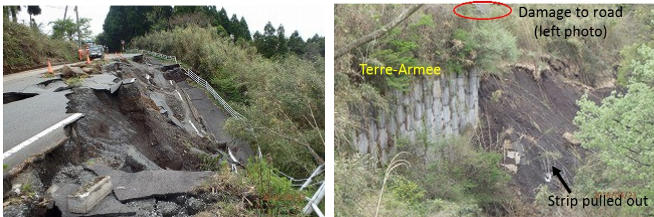
Figure 35. Damage to road embankment and reinforced retaining wall (Terre-Armee) (site 22 in Fig. 26) ( 32^{\circ} 52'52.01''N , 131^{\circ} 00'14.84''E ).
