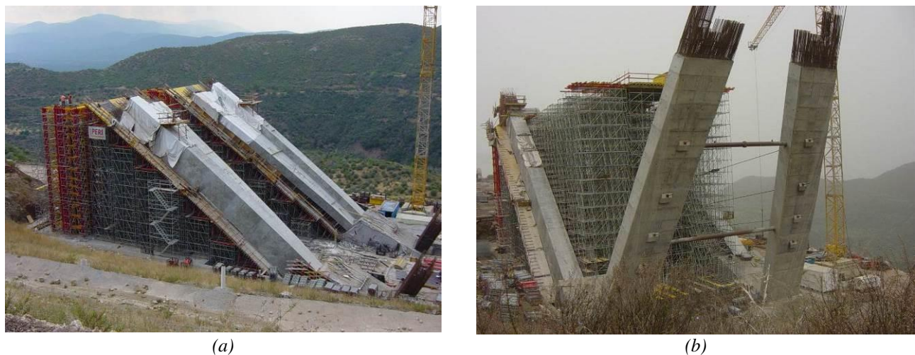
Figure 9. Construction of the (a) curved struts and (b) straight struts of the bridge pier.
