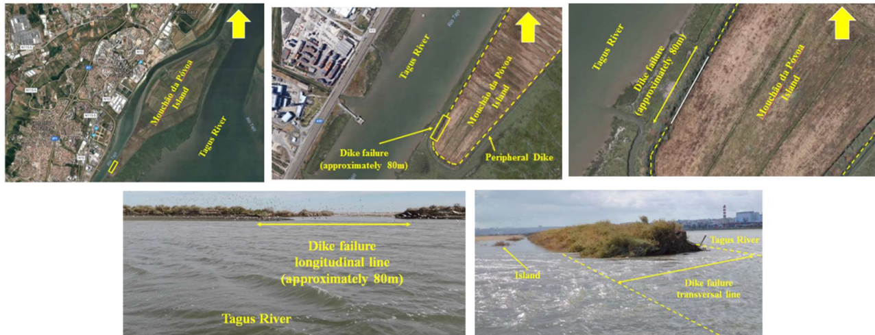
Figure 38. Location and view of the dike failure.
