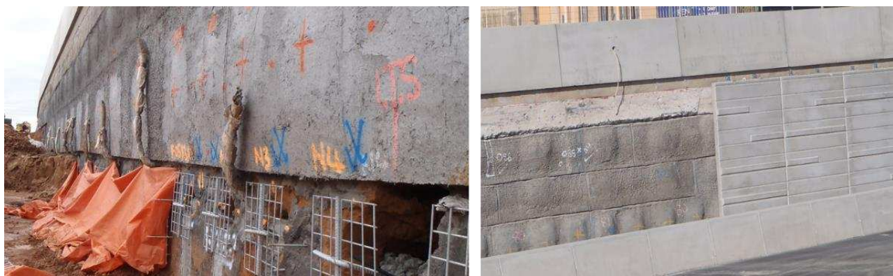
Figure 11. Photographs of wall prepared for shotcreting (left) and shotcreting completed with some facing panels installed (right).
