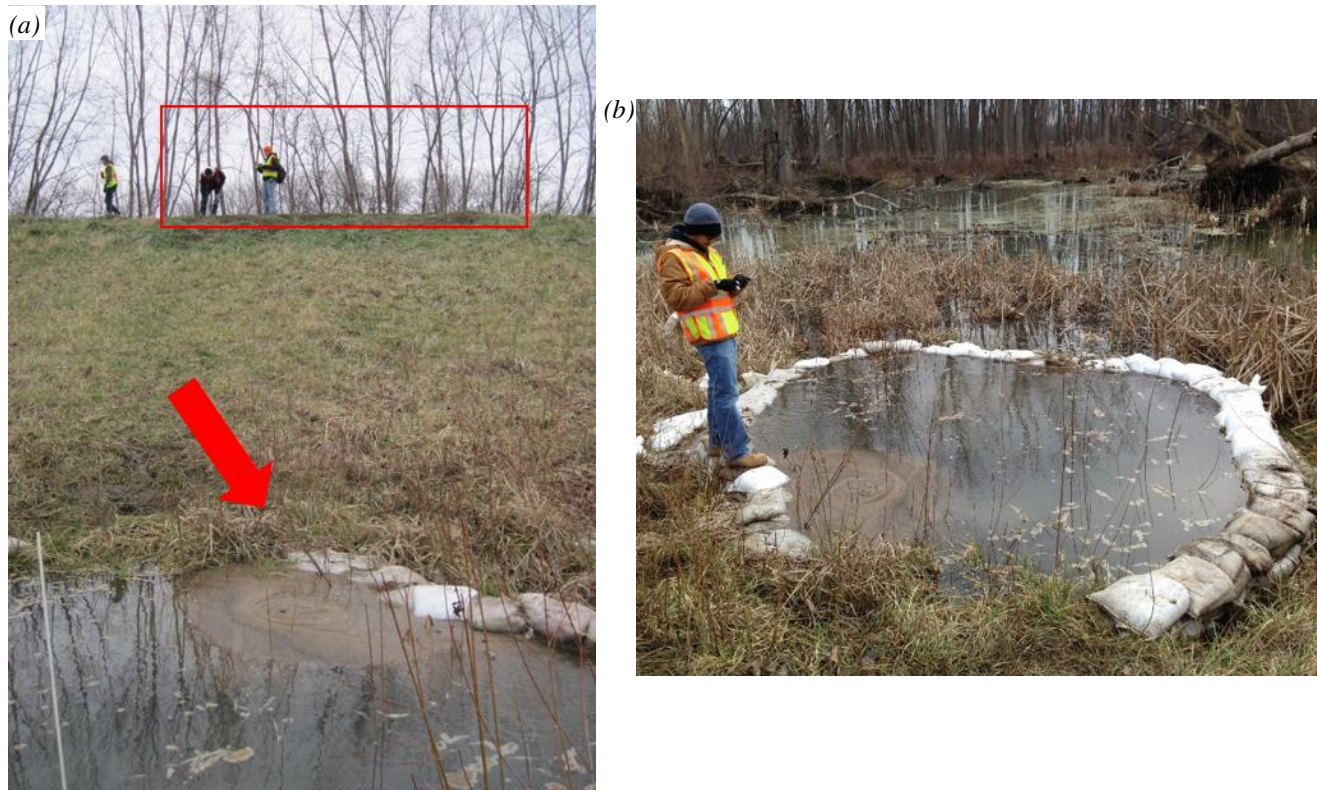
Figure 5. December 2015 flood reconnaissance: (a) settlement of crown with active sand boil at toe of levee, (b) active sand boil with sand bag ring (Rutherford et al. 2016).
