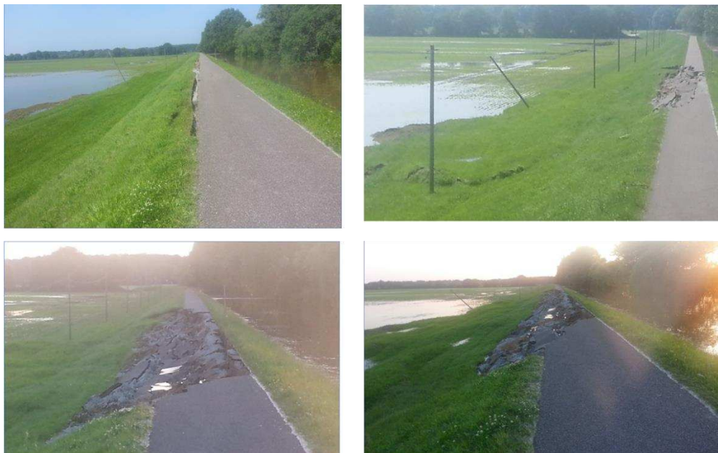
Figure 6. Photo series over time (upper left: 08.06.2013-10:37, initial break at the edge of the slope, upper right: 08.06.2013-14:10, horizontal shifts, bulge of the toe, lower left: 08.06.2013-20:51 continuing failure, lower right, 08.06.2013-20:55, continuing failure with the visual predictors (Grubert, 2013). Riverside of the levee is on the right for all photos.
