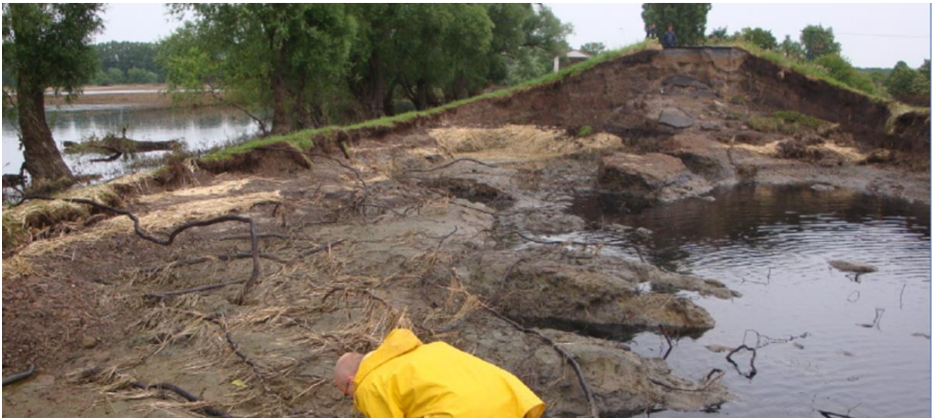
Figure 7. Photo of the cross-section of the breached levee (Grubert, 2013).
