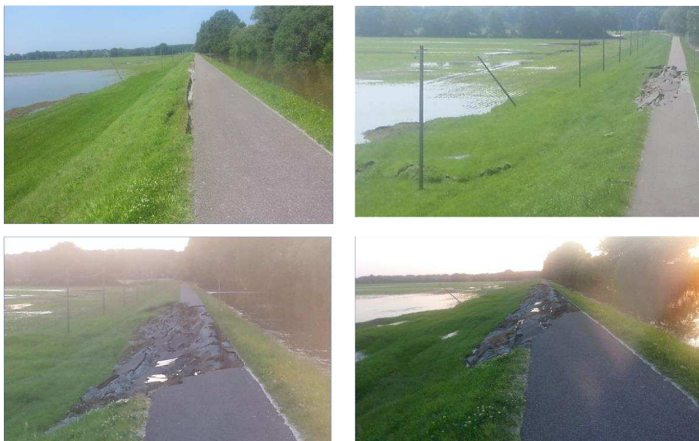
Figure 6. Photo series over time (upper left: 08.06.2013-10:37, initial break at the edge of the slope, upper right: 08.06.2013-14:10, horizontal shifts, bulge of the toe, lower left: 08.06.2013-20:51 continuing failure, lower right, 08.06.2013-20:55, continuing failure with the visual predictors (Grubert, 2013). Riverside of the levee is on the right for all photos.
