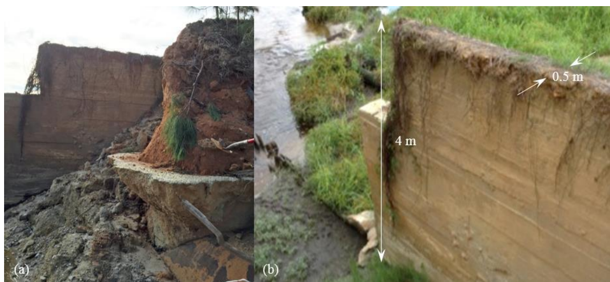
Figure 23. Concrete wall in the upstream section of Dam C, next to the breach zone: a) southwest view from downstream, and b) southeast view from crest of dam.
