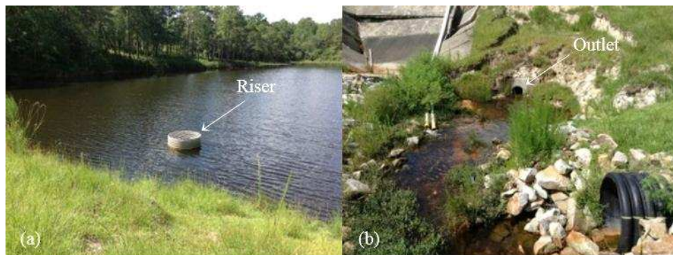
Figure 27. Primary spillway in Dam D: a) riser structure (southwest view from crest); and b) outlet pipe (southwest view from downstream).
