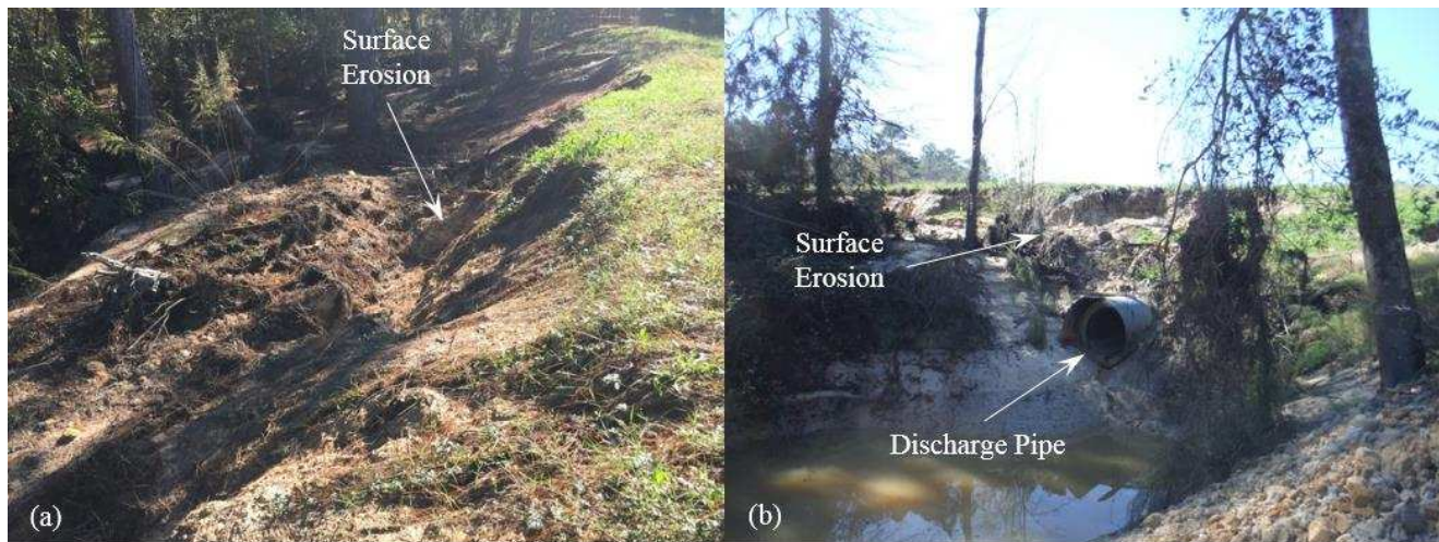
Figure 16. Surface erosion on downstream side slope of Dam B: a) south view from the crest of dam and b) west view from downstream.
