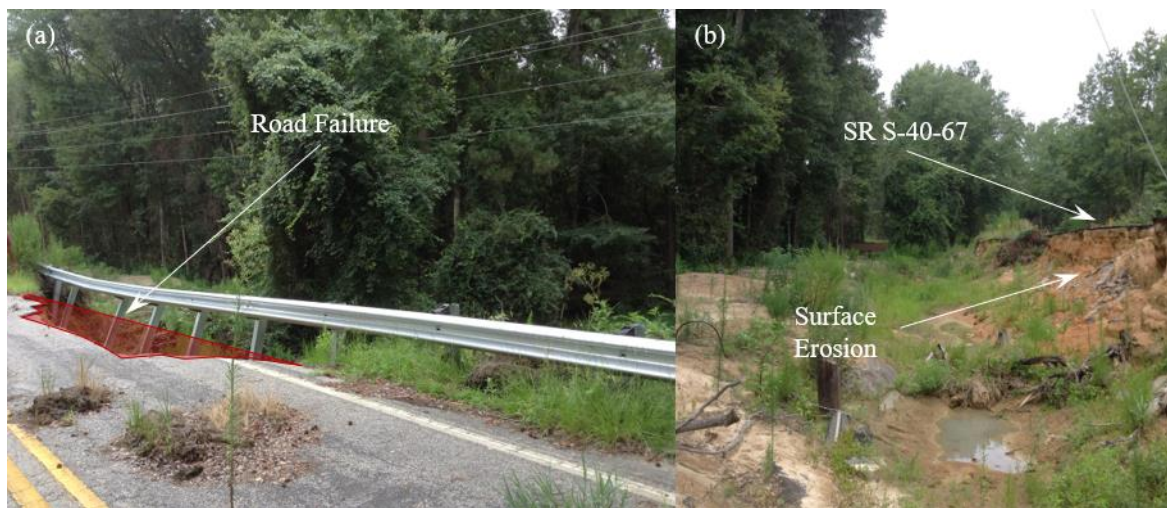
Figure 7. Failure of Dam A: (a) road failure of State Road S-40-67 (southeast view from S-40-67), and (b) surface erosion due to overtopping (west view from downstream).
