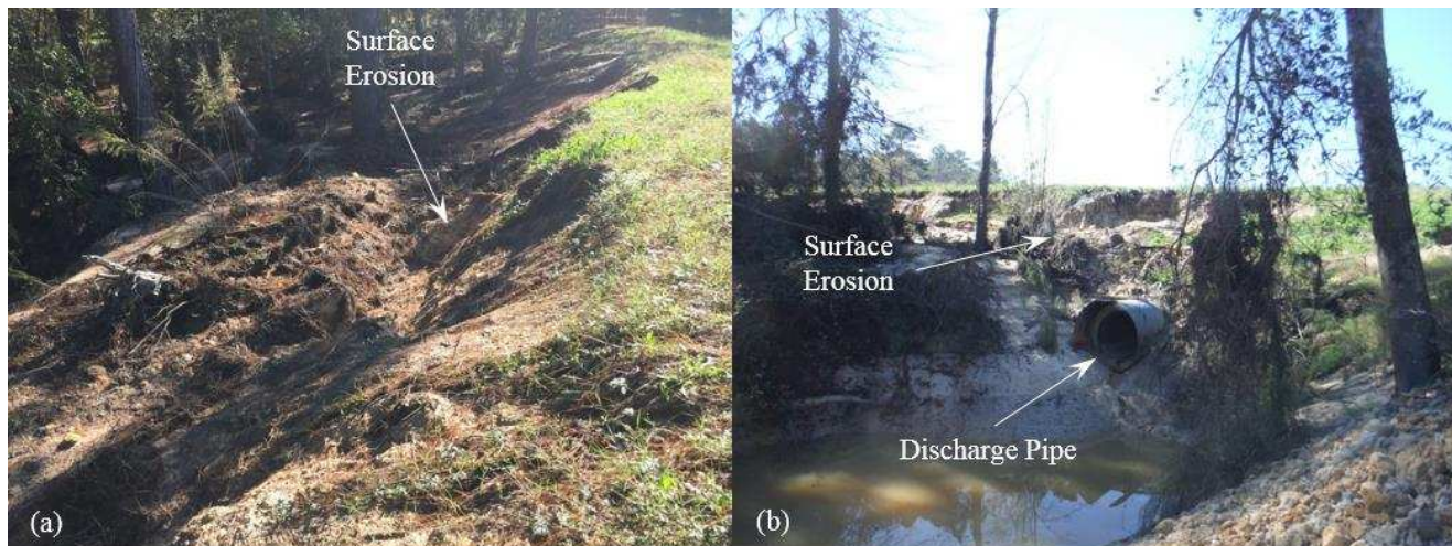
Figure 16. Surface erosion on downstream side slope of Dam B: a) south view from the crest of dam and b) west view from downstream.
