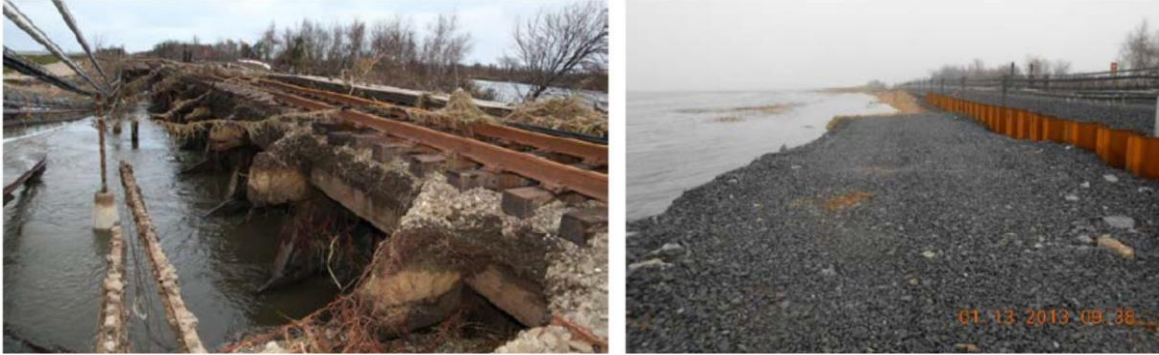
Figure 16. Earth embankment washouts in Queens, along Rockaway subway [A] line after Sandy with old LIRR infrastructure exposed (left) and post mitigation work (right). Photos by Khinda, ed. (2013).
