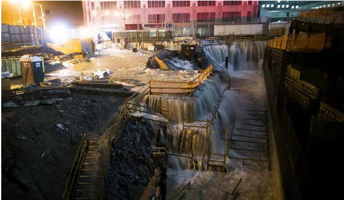
Figure 14. Open excavation flooding at the World Trade Center site (Photo: Associated Press).
