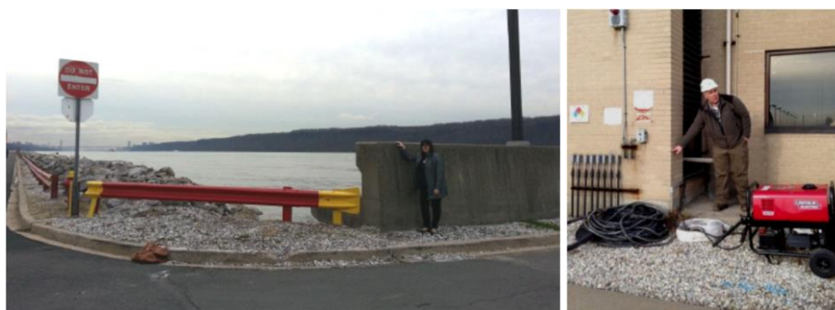
Figure 27. Yonkers Joint WWTP: junction of rip-rap revetment and seawall, looking south (left); vent grates in aeration blower building where water entered, with flood water elevation shown by plant superintendent (right); GEER (2014).
