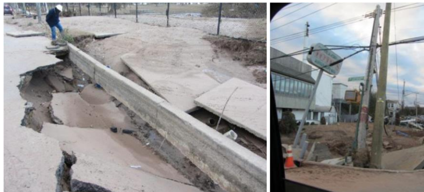
Figure 24. Scour undermining of street and utilities at Seaview Blvd, SI (40.579283°N, 74.077849°W, 11/4/12, GEER, 2014).
