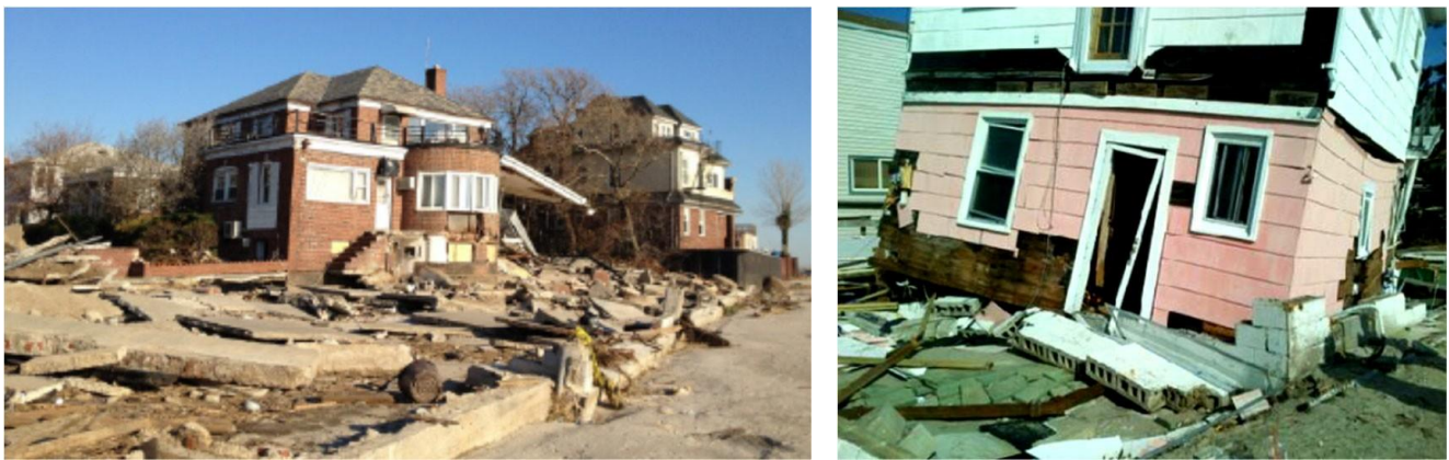
Figure 20. Undermining of beachfront retaining wall and loss of retained soil, Sea Gate, Brooklyn (left, 11/9/12); Destroyed CMU wall foundation, Breezy Point, Queens (right, 11/12/12). Photos by NYCDob (GEER, 2014).
