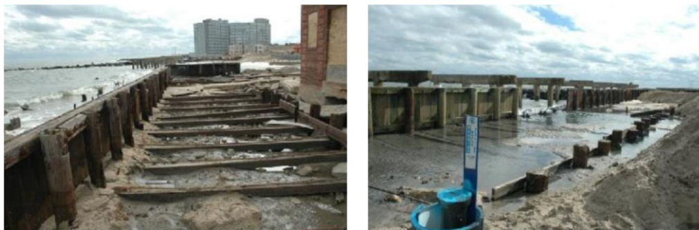
Figure 25. Bulkhead in Atlantic City, NJ: backfill soil washed away, exposing severely corroded tie rods (GEER, 2014).
