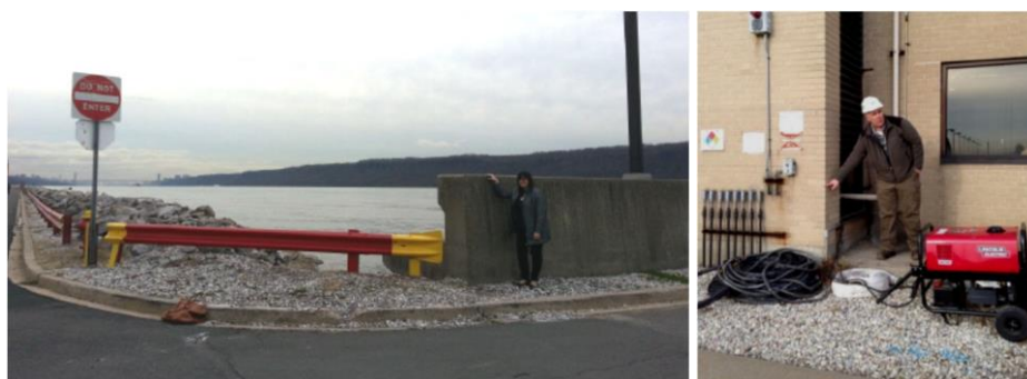
Figure 27. Yonkers Joint WWTP: junction of rip-rap revetment and seawall, looking south (left); vent grates in aeration blower building where water entered, with flood water elevation shown by plant superintendent (right); GEER (2014).
