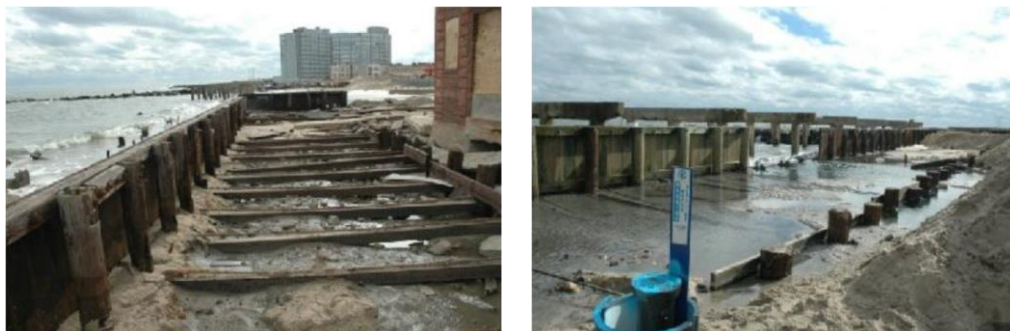
Figure 25. Bulkhead in Atlantic City, NJ: backfill soil washed away, exposing severely corroded tie rods (GEER, 2014).
