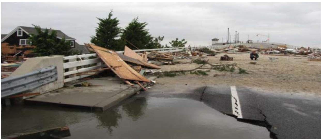
Figure 10. Foundation undermining at east abutment of Mantoloking Bridge ( 40.040058^{\circ}\text{N} , 74.051886^{\circ}\text{W} ; GEER, 2014).
