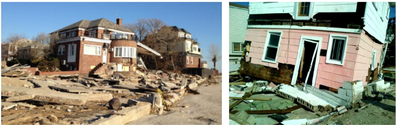
Figure 20. Undermining of beachfront retaining wall and loss of retained soil, Sea Gate, Brooklyn (left, 11/9/12); Destroyed CMU wall foundation, Breezy Point, Queens (right, 11/12/12). Photos by NYCDob (GEER, 2014).
