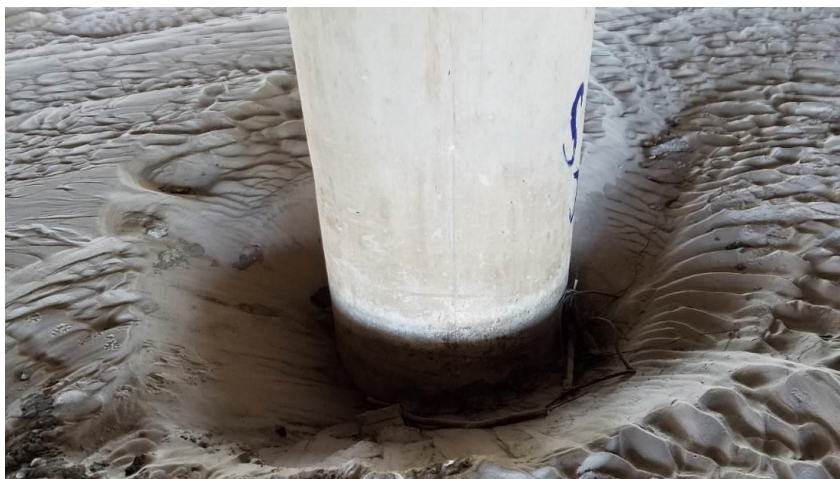
Figure 40. Scour around columns on San Jacinto Banks (sandy soil). The scour hole was approximately 2.4 m (8 ft) across and 0.6 m (2 ft) deep (September 11, 2017, Time 10:59 CDT, 30.243364°N, 95.46452°W).
