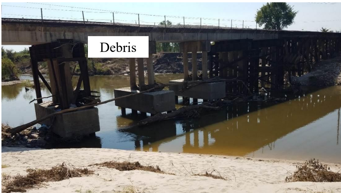
Figure 42. Debris on railroad bridge indicating flow levels and scour around pile caps below current flow levels (September 11, 2017, Time 11:10 CDT, 30.24688° N, 95.45796° W).
