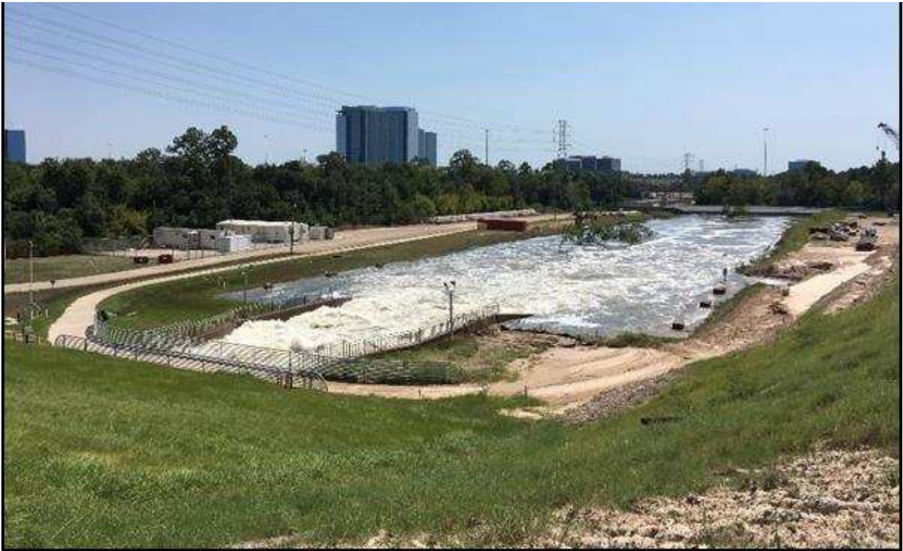
Figure 5. Addicks outlet releasing \sim 170 \text{ m}^3/\text{s} ( \sim 6000 \text{ cfs} ) (September 9, 2017, 29.79026^\circ \text{ N} , 95.62378^\circ \text{ W} ).
