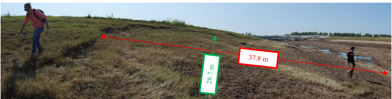
Figure 18. Ditch H levee, dimensioned slope failure (September 10, 2017, 29.55797°N, 95.63792°W).
