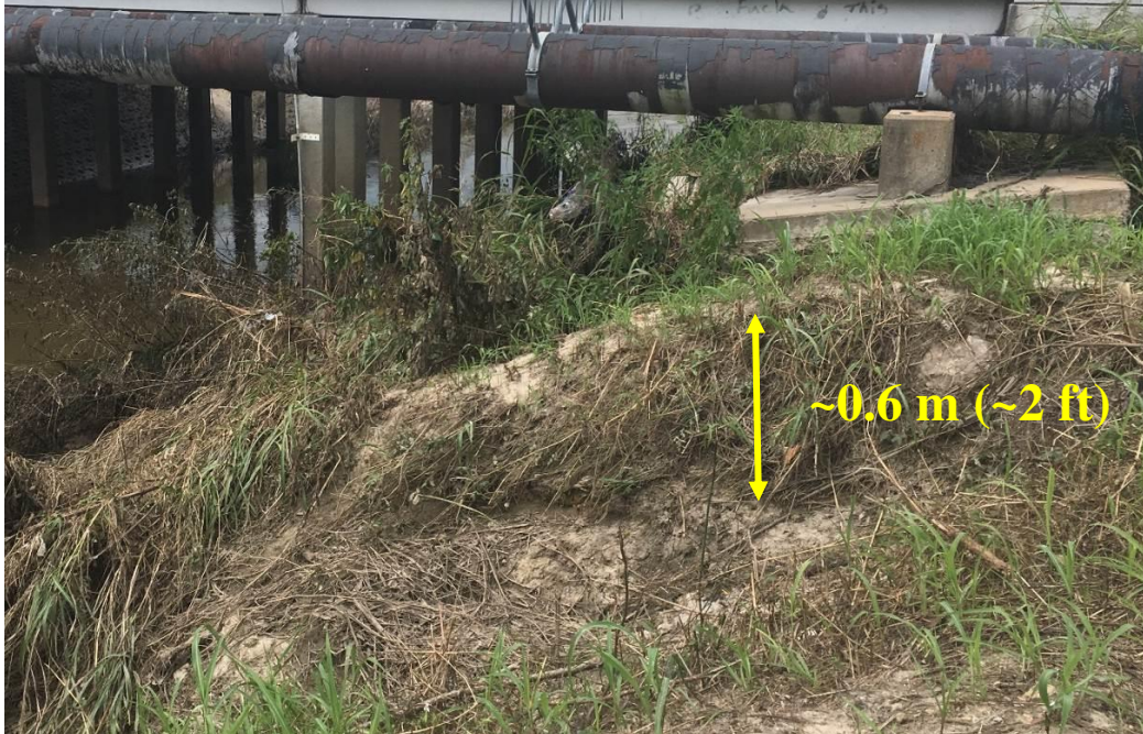
Figure 44. Shallow soil failure along the north bank of Mustang Bayou, adjacent to pipe-support foundation (September 4, 2017, Time 12:48 CDT, 29.40889° N, 95.23234° W).
