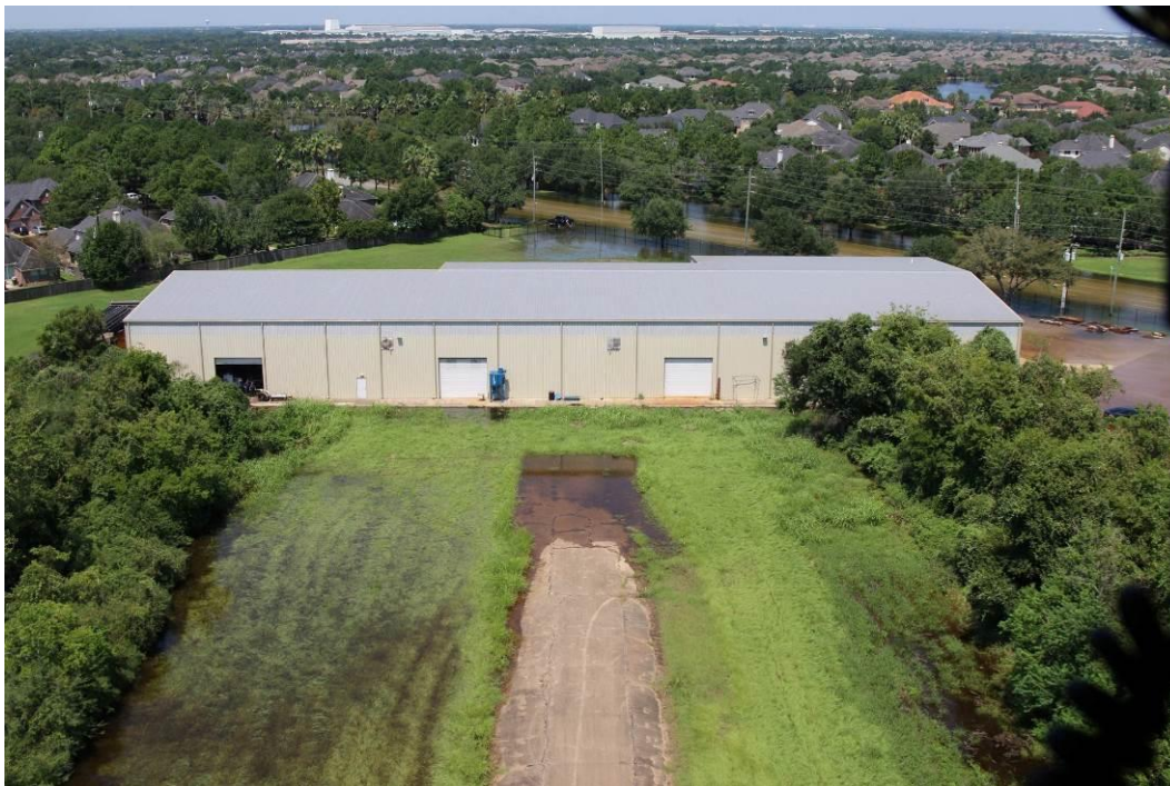
Figure 8. North end of Addicks auxiliary spillway (September 3, 2017, 29.84977° N, 95.58904° W, photo by USACE).
