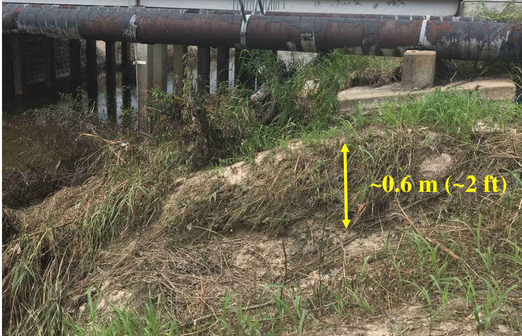
Figure 44. Shallow soil failure along the north bank of Mustang Bayou, adjacent to pipe-support foundation (September 4, 2017, Time 12:48 CDT, 29.40889° N, 95.23234° W).
