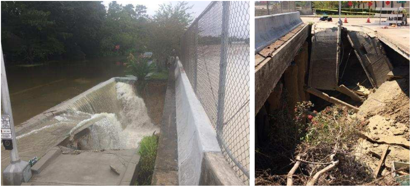
Figure 32. Damage of the walkway slab on Beltway 8 (left photo courtesy Brian Klein, a resident in the area, August 27, 2017, and right photo courtesy of a construction worker on site, 29.76735° N, 95.56219° W).
