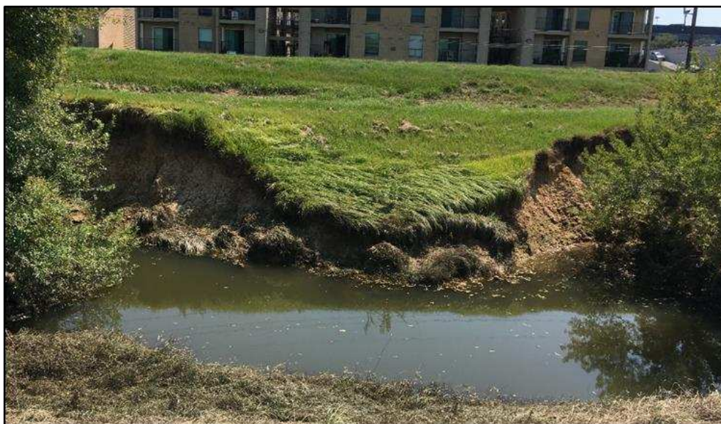
Figure 12. Slope failures along Turkey Creek drainage ditch (September 9, 2017, 29.79009° N, 95.59639° W).
