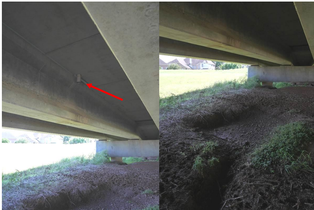
Figure 20. Erosion on Ditch H levee under the University Blvd Bridge due to flow impact from bridge drainage outfall (red arrow, September 10, 2017, 29.55902° N, 95.63744° W).
