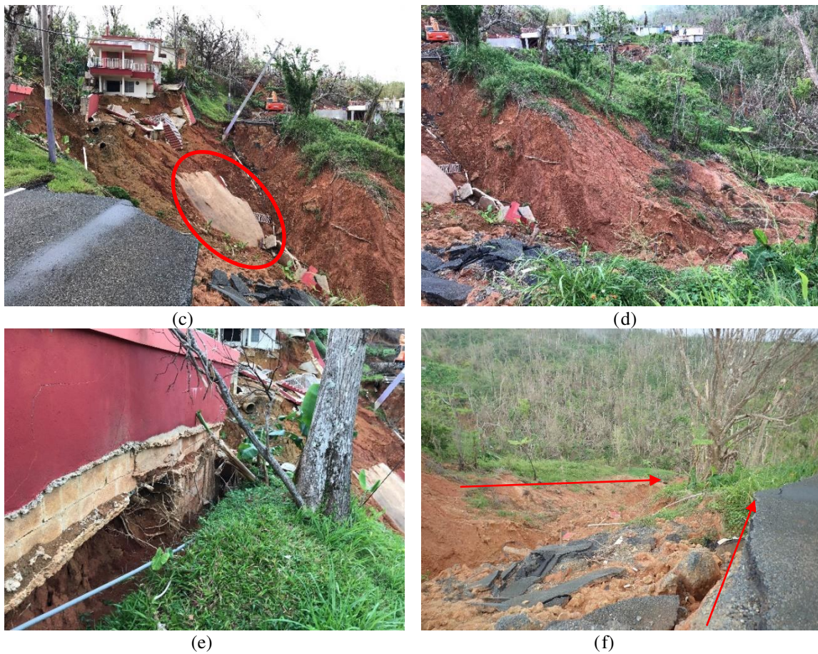
Figure 23. Road failure affecting PR-186 (GEER mission Site 7; Silva-Tulla et al., 2018).
