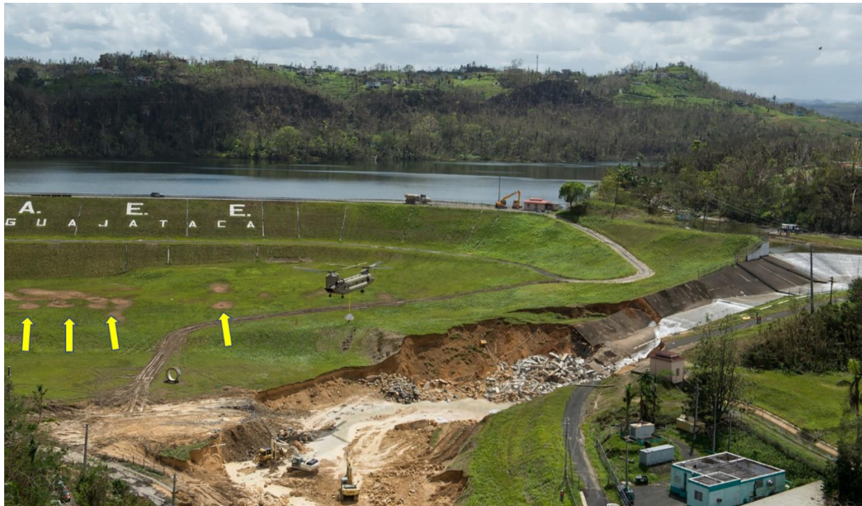
Note: Yellow arrows show location of apparent sand boils downstream of the dam toe.
