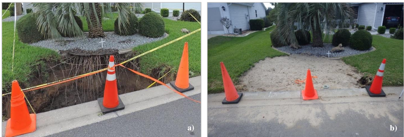
Figure 7. Sinkhole at 2532 Botello Avenue at 28°57'10.60"N latitude and 81°59'30.50"W longitude: a) prior to repair (Villages News 2017), b) following repair (Hudyma et al., 2017).
