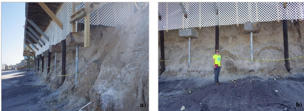
Figure 10: Erosion undercutting both the timber pile supports and micropile supported concrete footings for a beach house with continued slope failures in drying sand at 29°56'47.00"N latitude and 81°18'8.10"W longitude after Hurricane Irma.
