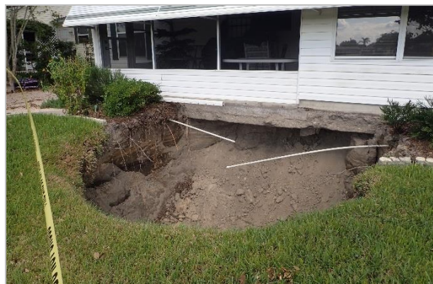
Figure 6. Sinkhole undercutting a foundation at 2536 Botello Road at 28^{\circ}57'11.67''N latitude and 81^{\circ}59'30.05''W longitude (Hudyma et al., 2017).
