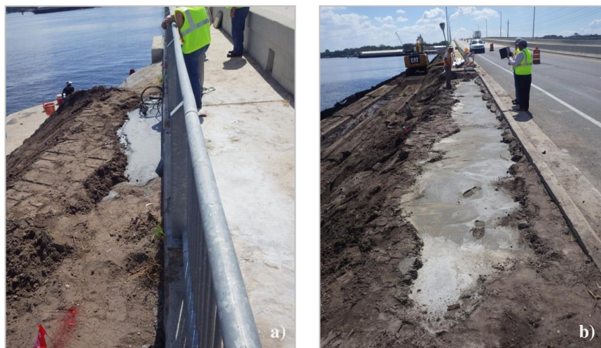
Figure 23: Repaired northeastern bridge embankment for US 17 bridge over the Trout River at 30°23'45.44"N latitude and 81°38'53.95"W longitude that includes the rebuilt soil and excavatable flowable fill trench embankment (a) adjacent to the concrete covered, stacked concrete sack wall; and (b) roadway edge (Hudyma et al., 2017).
