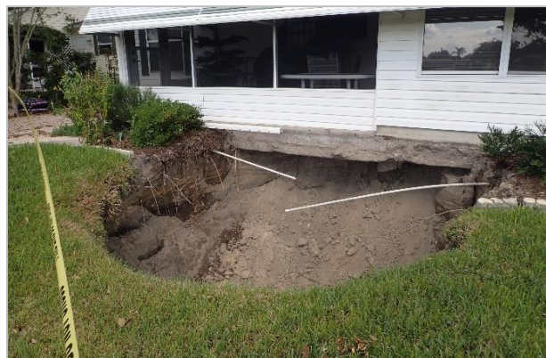
Figure 6. Sinkhole undercutting a foundation at 2536 Botello Road at 28^{\circ}57'11.67''N latitude and 81^{\circ}59'30.05''W longitude (Hudyma et al., 2017).
