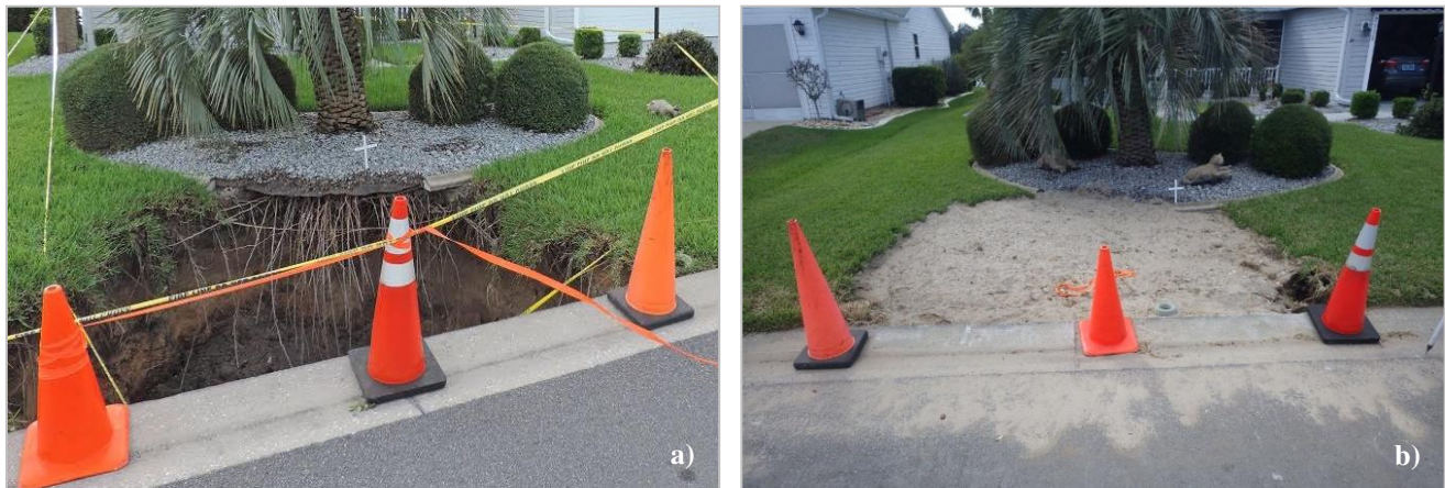
Figure 7. Sinkhole at 2532 Botello Avenue at 28°57'10.60"N latitude and 81°59'30.50"W longitude: a) prior to repair (Villages News 2017), b) following repair (Hudyma et al., 2017).
