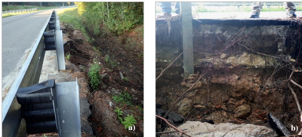
Figure 17: Erosion damage of the northern section of Lake Hampton Road at the Pigeon River crossing north of the dam near 30°46'45.19"N latitude and 81°58'24.6"W longitude.
