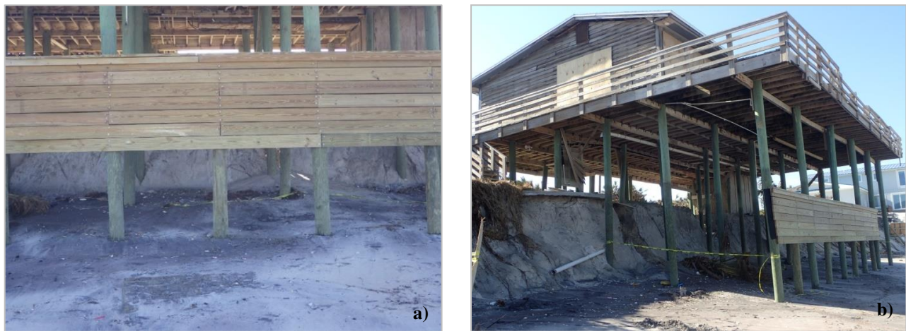
Figure 11. (a) Shallowly embedded timber seawall at approximately 29^{\circ}56'49.30''N latitude and 81^{\circ}18'9.37''W longitude, showing significant erosion (about 2 m or 6.6 ft) below a residential structure; and (b) subsequent beach erosion and removal of the first story walls by wind and water.
