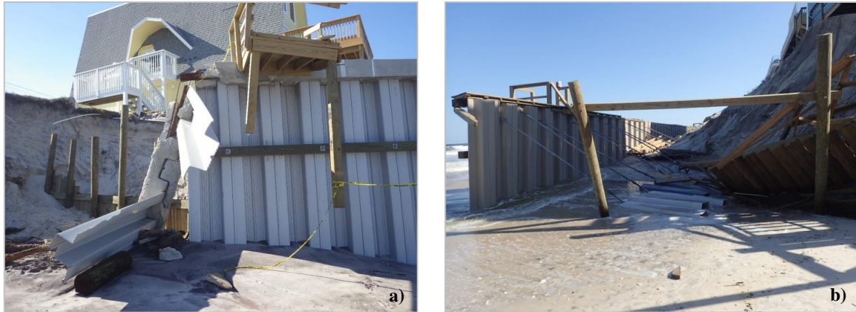
Figure 13: Failure of two residential sheet pile retaining walls from side erosion following Hurricane Irma, showing: (a) a partial sheet pile wing wall that was extended into the dune using timber piles and wooden lagging at 29^{\circ}56'55.10''N latitude and 81^{\circ}18'13.49''W longitude, and (b) the backside of the wall and anchors from the side where the wing wall was not yet installed at 29^{\circ}56'46.05''N latitude and 81^{\circ}18'7.5''W longitude (Hudyma et al., 2017).
