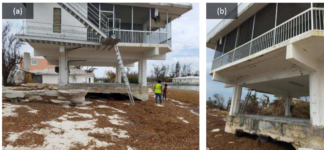
Figure 15. (a) The foundation of an elevated home was undermined due to scouring around the structure; (b) a close-up view shows damage to the structural integrity of the home (collected September 26, 2017; location 24^{\circ}41'31.86''N , 81^{\circ}4'57.29''W ).
