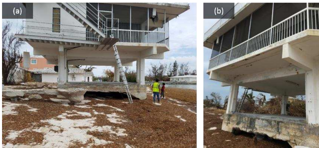
Figure 15. (a) The foundation of an elevated home was undermined due to scouring around the structure; (b) a close-up view shows damage to the structural integrity of the home (collected September 26, 2017; location 24^{\circ}41'31.86''N , 81^{\circ}4'57.29''W ).
