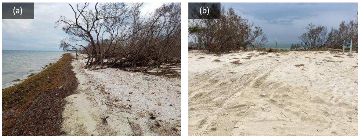
Figure 18. (a) The beach width was narrowed due to erosion and algae washed up on the beach, and (b) sediment approximately 0.3 m in depth was deposited in the beach access area (collected September 26, 2017; location 24^{\circ}43'48.42''N , 81^{\circ}0'5.81''W ).
