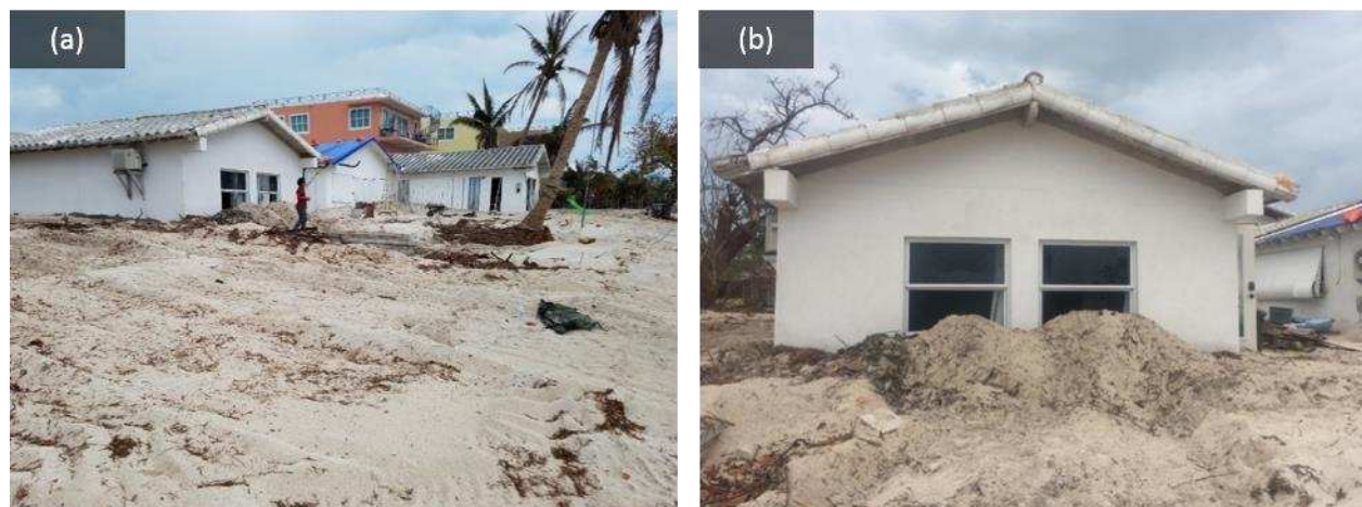
Figure 13. (a) Large volumes of sediment were deposited around houses and other structures and (b) buried them with approximately 1 m of sand, reaching the bottom of window sills (collected September 26, 2017; location 24°41'31.52"N, 81°4'56.31"W).
