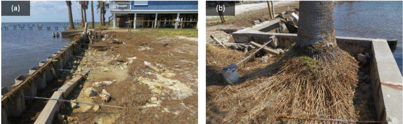
Figure 6. (a) Supporting steel rods were exposed after storm surge retreat scoured the backside of a bulkhead, and (b) scour was also observed around other fixed objects (collected September 3, 2017; location 28^{\circ}10'11.24''N , 97^{\circ}1'2.03''W ).
