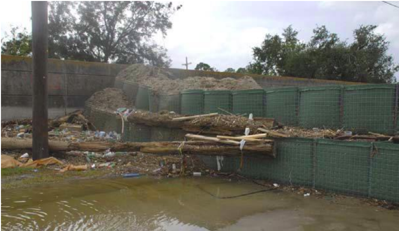
Figure 31. End of temporary bin wall at tie-in to I-Wall, post-Gustav (September 2008, 30.0122° N, 90.0313° W, http://www.mvn.usace.army.mil/HPS/Status%20Report%20Newsletters/Sept_9_2008.pdf )
