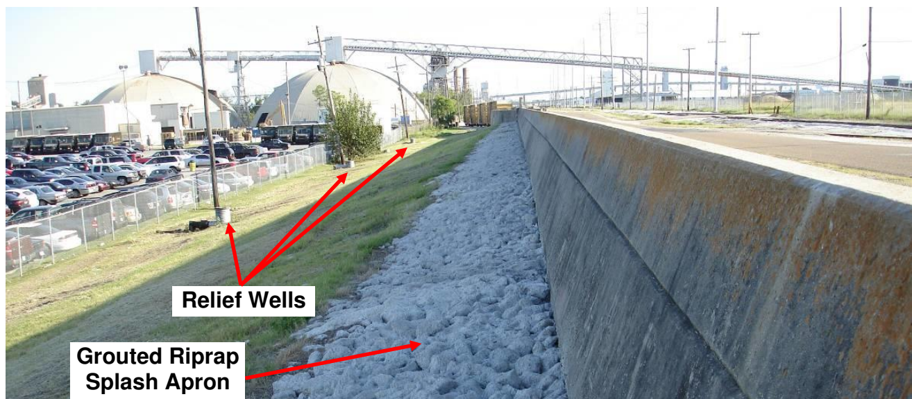
Figure 28. IHNC floodwall near East Morrison Road. Note splash apron (center) and relief wells (left). (October 2, 2008, 30.0248° N, 90.0295° W)
