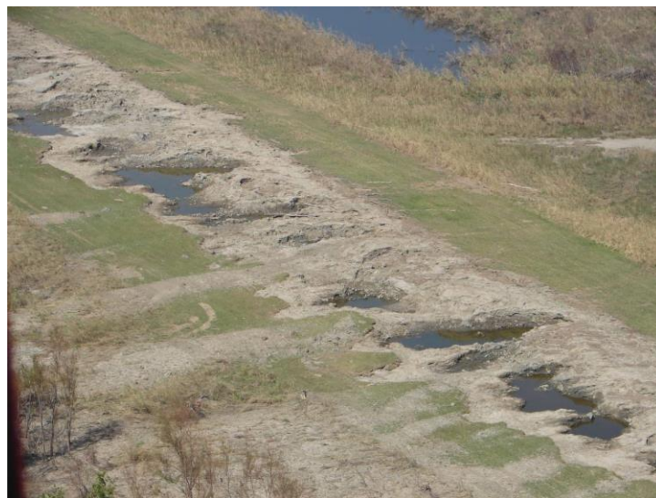
Figure 11. Post-Katrina MRGO frontage levee. (October 14, 2005, ~89.8° W, ~29.9° N, L. Harder)
