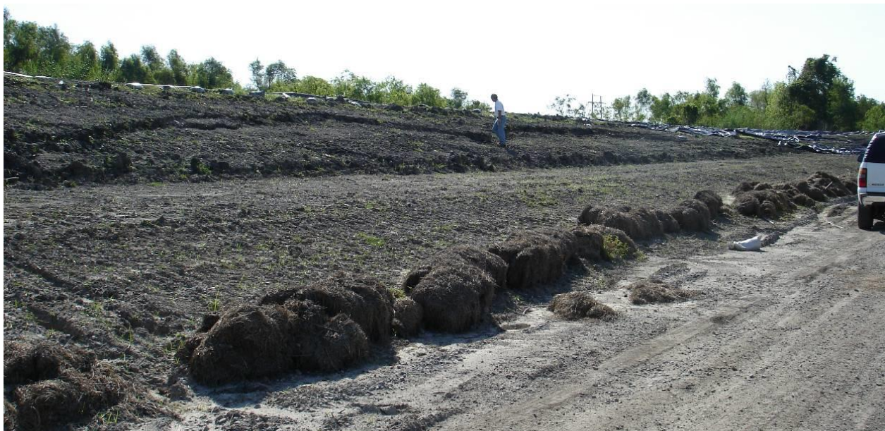
Figure 35. Protected side slope of the Plaquemines Parish back levee and slide. (October 3, 2008, 29.8506° N, 89.9085° W)
