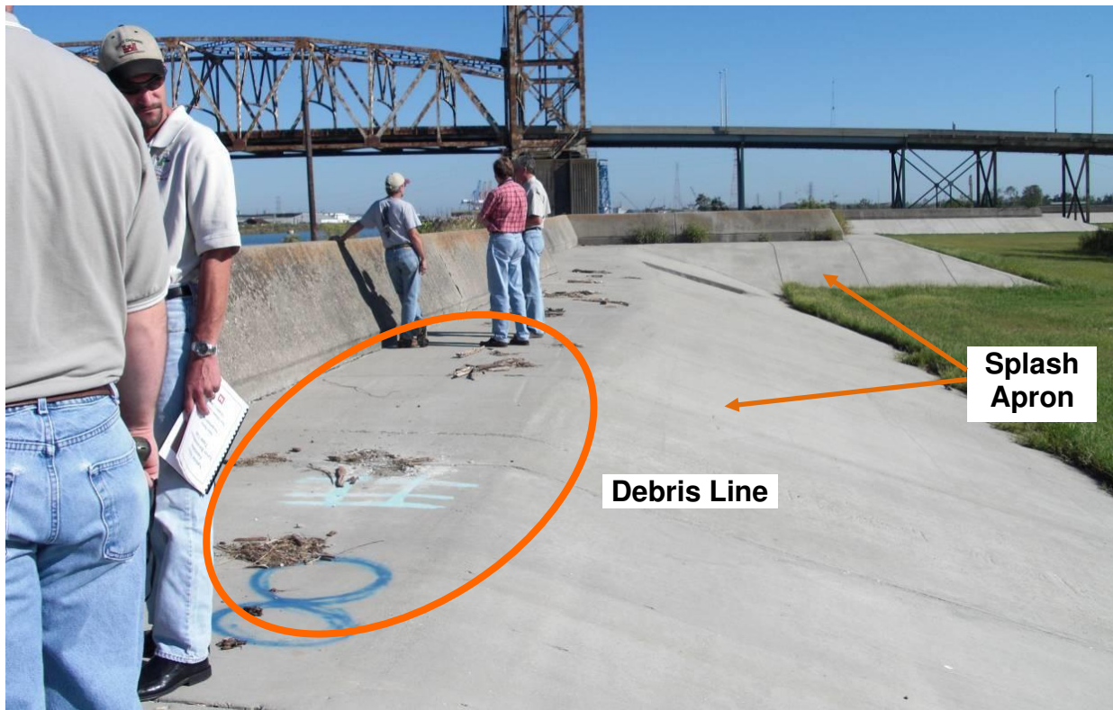
Figure 26. Hardened I-wall along east side of the IHNC south of Claiborne Avenue looking north (IHNC is to the left and Lower 9 th Ward / Holy Cross to the right). (Oct. 2, 2008, 29.9682° N, 90.0250° W)
