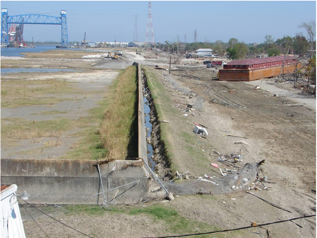
Figure 24. Post-Katrina IHNC East floodwall with southern-most breach and the scour, looking north, from the Claiborne Avenue Bridge. (October 11, 2005, 29.9685° N, 90.0238° W, L. Harder)
