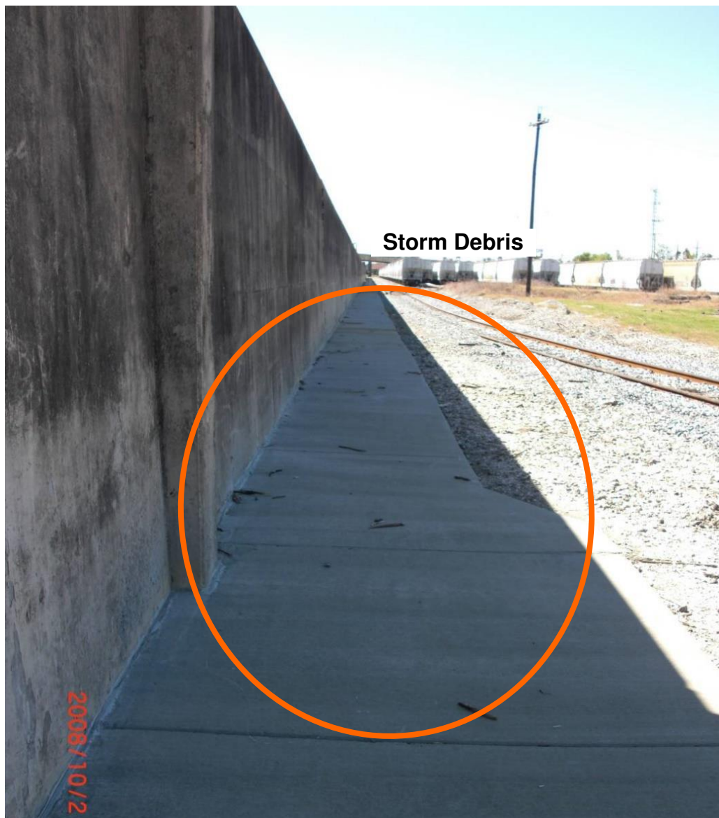
Figure 23. Photograph from October 2, 2008, of IHNC West T-wall (same section as shown during Gustav in Figures 20 and 21). (October 2, 2008, 29.970° N, 90.026° W)
