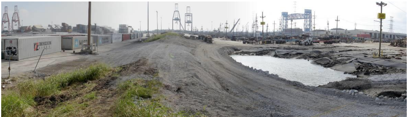
Figure 16. Post-Katrina IHNC West levee breach site, October 2005 (The breach had been temporarily repaired; note scour hole). (October 4, 2005, 29.9880° N, 90.0263° W, L. Wooten)
