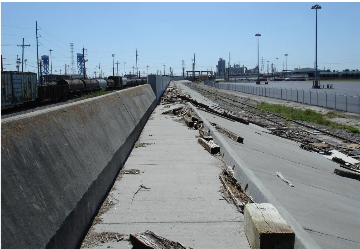
Figure 6. I-wall and splash apron, IHNC west along France Road; new L-wall and splash apron in background. (October 2, 2008, 90.0272° W, 90.0272° W)
