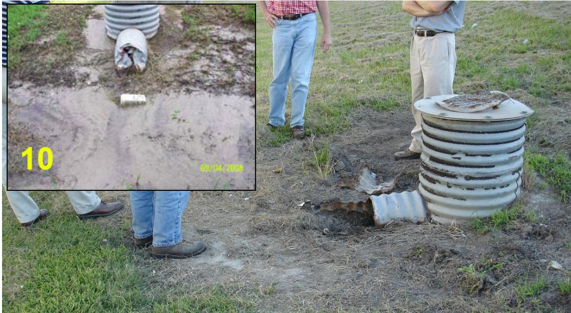
Figure 29. Relief well cover, as of October 2008, with inset taken from the USACE Hurricane Gustav Damage Assessment Team SITREP on September 5, 2008. (October 2, 2008, 30.0249° N, 90.0294° W)
