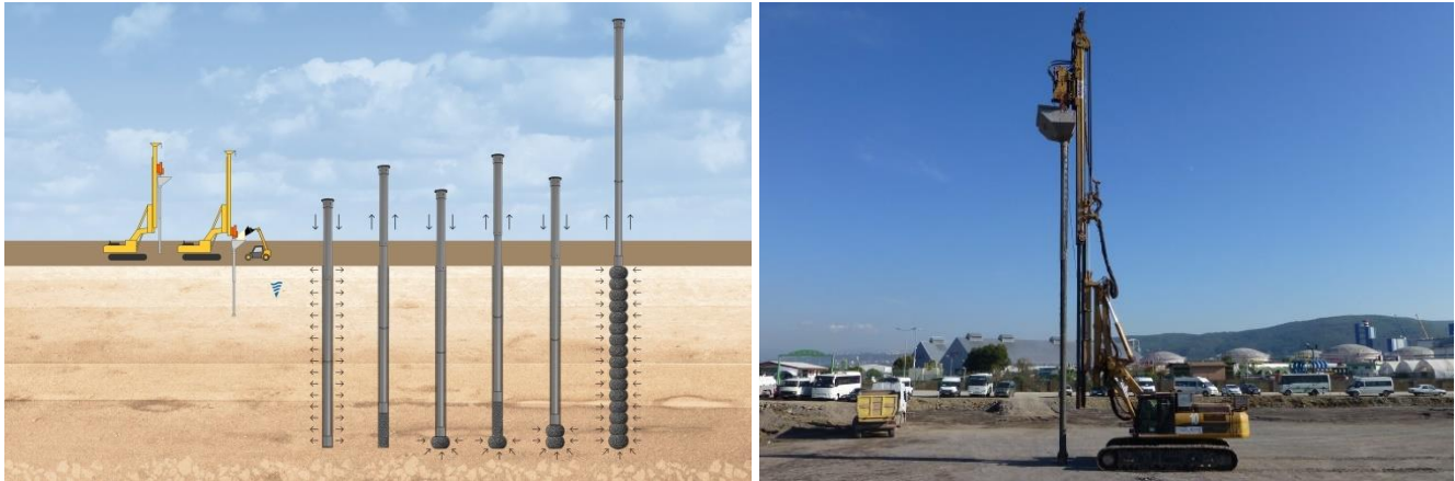
Figure 8. Construction methodology of RAP Impact elements and a view from the field construction.
