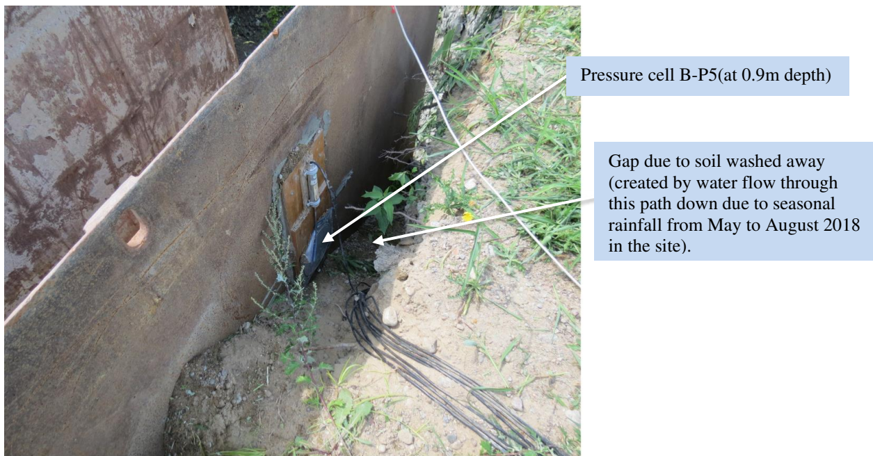
Figure 21. Surrounding soil washed away by heavy rainfall affecting pressure cell at 0.9 m.
