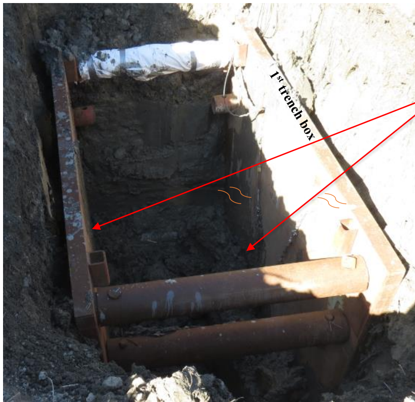
Figure 23. Likely “fixed end condition” developed at the lower end of the first trench box due to 300 mm insertion into the soil.
