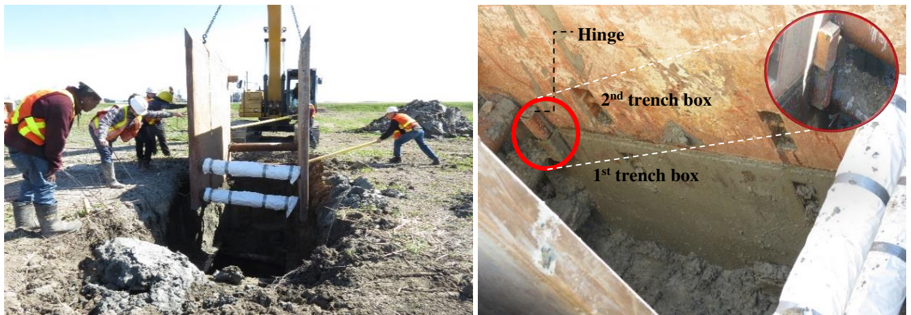
Figure 12. Second (upper) trench box is being placed on top of the first (lower) box in the trench.
