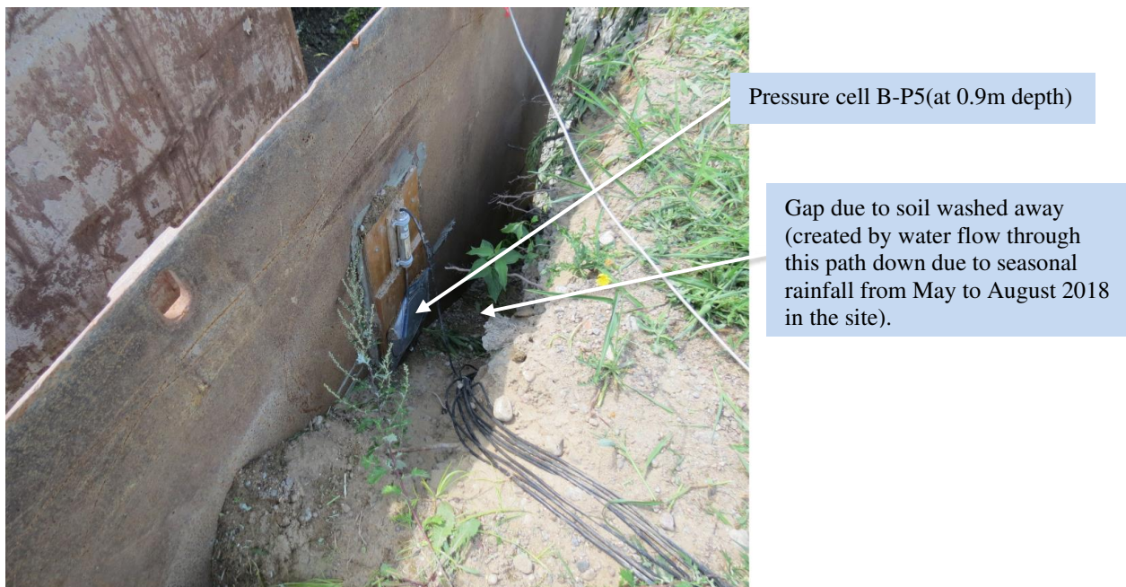
Figure 21. Surrounding soil washed away by heavy rainfall affecting pressure cell at 0.9 m.
