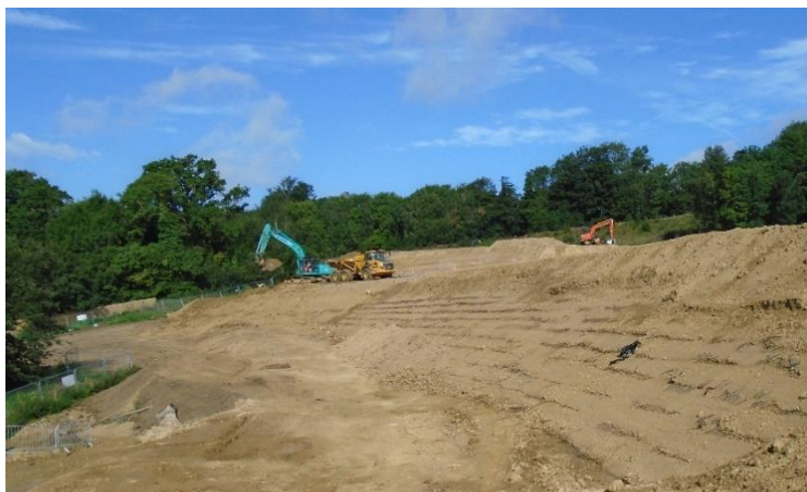
Figure 5. Shallow slope during construction at the Queenway Gateway Link project where the drainage geogrids are placed in layers at equidistance vertical centers; the facing element of the slope will be created using hydro seeding over an erosion geosynthetic mat.
