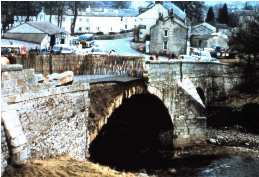
Figure 9. Failure of spandrel wall, Kettlewell New Bridge, 1984.
