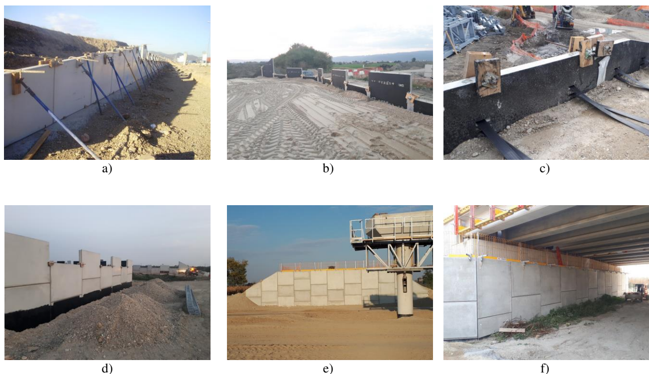
Figure 9. D4R7 Project VSoL ® reinforced soil bridge abutment construction stages: (a) 1 st panel row installation, (b) backfilling, (c) polymeric strips placement, (d) frontal embedment detail, (e) frontal view, and (f) bridge deck arrangement.
