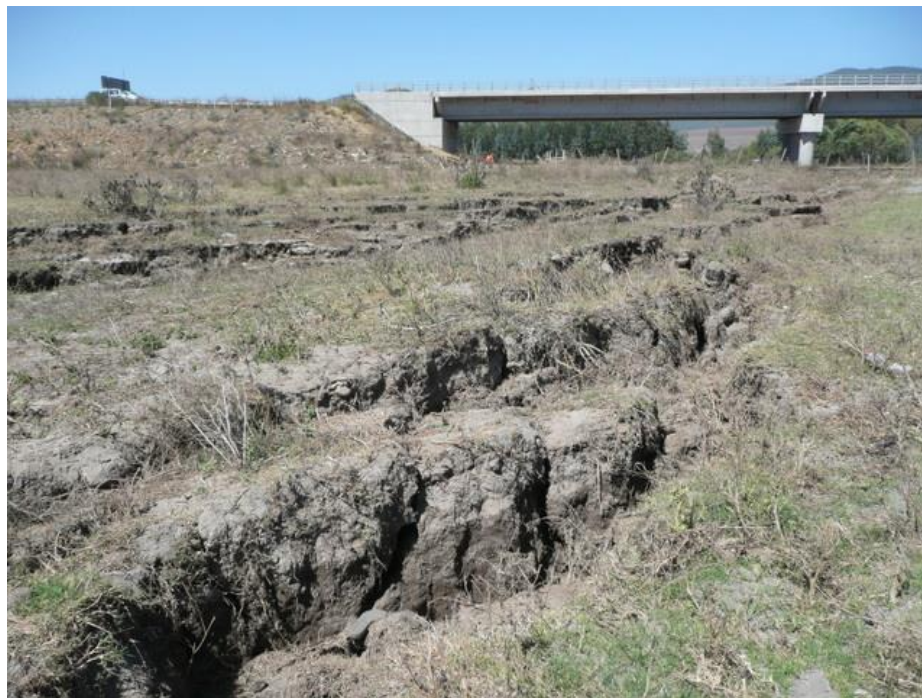
Figure 3. Lateral spreading at the north side of the bridge. Cracking showing roughly 0.6 m of vertical and 0.8 m of lateral displacement toward the river (Bray et al., 2010).
