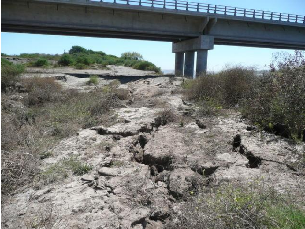
Figure 4. Liquefaction effects along the south side of the bridge (Bray et al., 2010).
