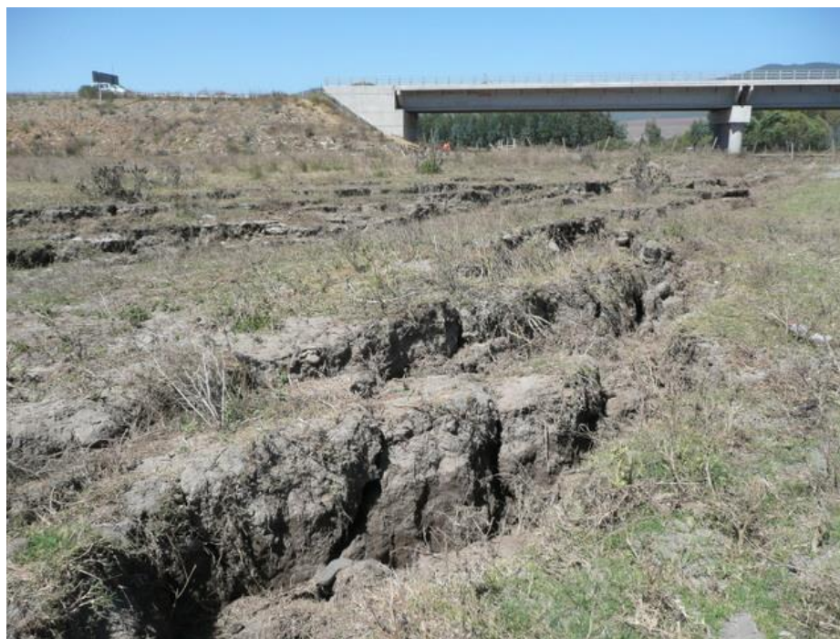
Figure 3. Lateral spreading at the north side of the bridge. Cracking showing roughly 0.6 m of vertical and 0.8 m of lateral displacement toward the river (Bray et al., 2010).
