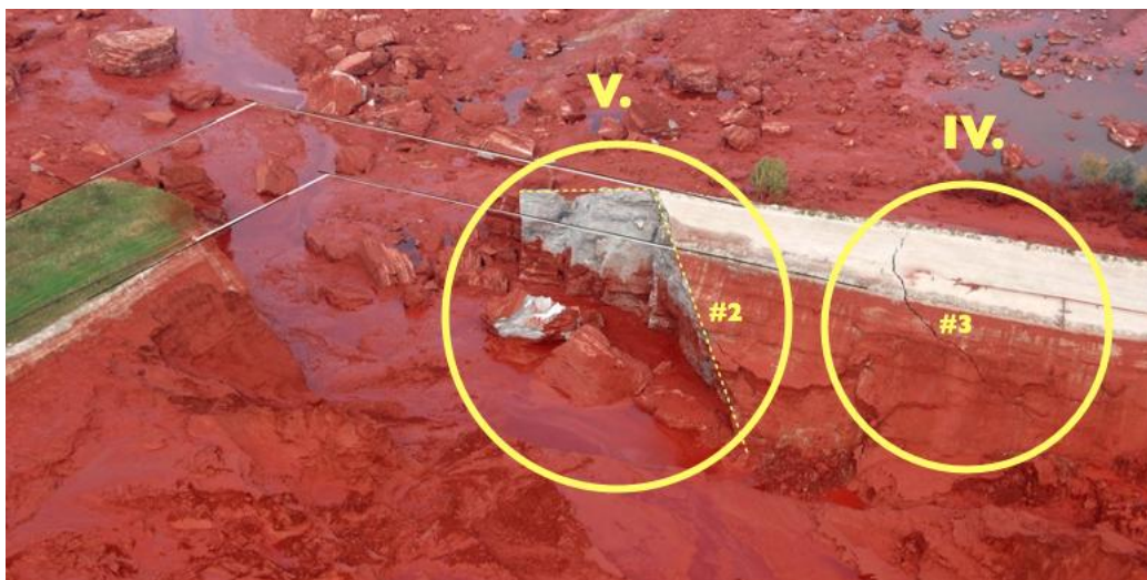
Figure 17. The fractures at Locations IV and V are hybrid fractures caused by the outflowing pressure of the red sludge and the additional settlement. These fractures occurred after the breach of the dam and they have no relevance to the failing of the dam. (Source: https://commons.wikimedia.org/wiki/File:Ajka_accident_d7df9fea08_b.jpg .)
