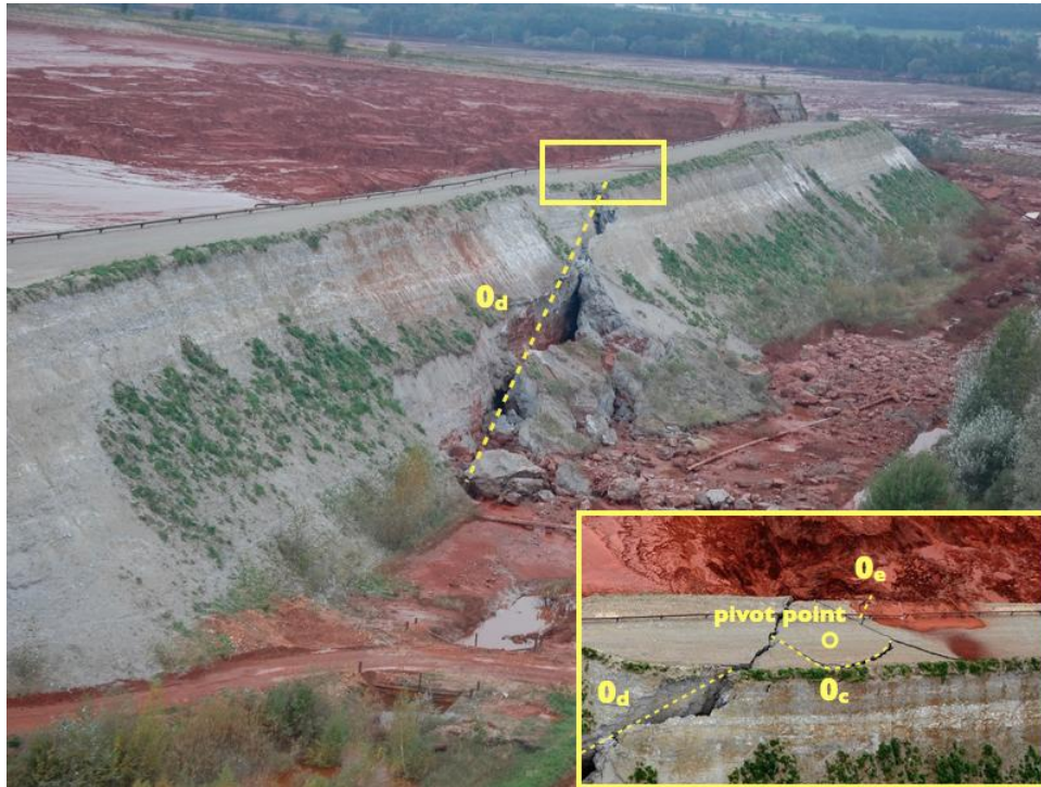
Figure 15. Shear fractures ( 0_c and 0_d ) caused by compressional stress at Location II are shown. These fractures were formed at the breach, resulting from the angular distortion of the failed dam section. On the opposite (reservoir) side, at the same time, extension fracture 0_b occurred (Figure 9), extending the existing fracture of -2_b . (Sources: https://www.nbcnews.com/slideshow/toxic-red-sludge-floods-towns-near-budapest-39514793 ; http://www.hungarianambiance.com/2011/09/possibility-of-act-of-terrorism-cant-be.html ).
