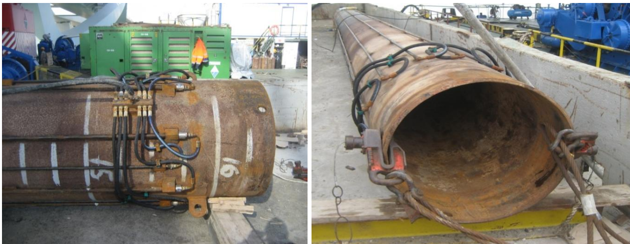
Figure 9. Distribution Lines on top of Casing Pile.
