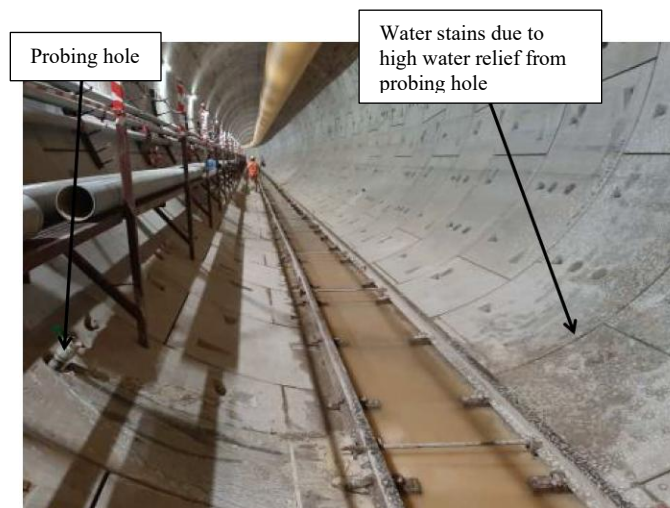
Figure 11. Observation of high water seepage through temporary tunnel probing.
