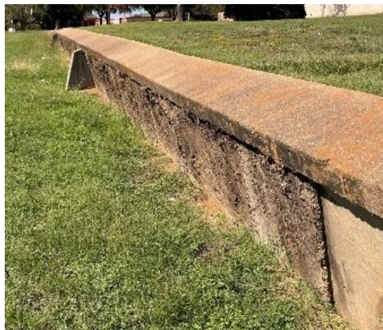
Figure 22. Wall retaining swelling soil with long-term inundation by a lawn watering system.
