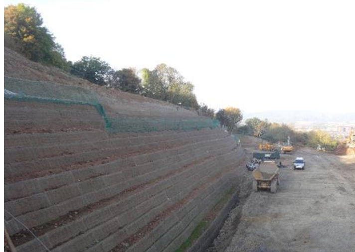
Figure 2. 17 m high structure constructed from draining geogrid and site won fill, Palmerston Park, Devon, October 2016.
